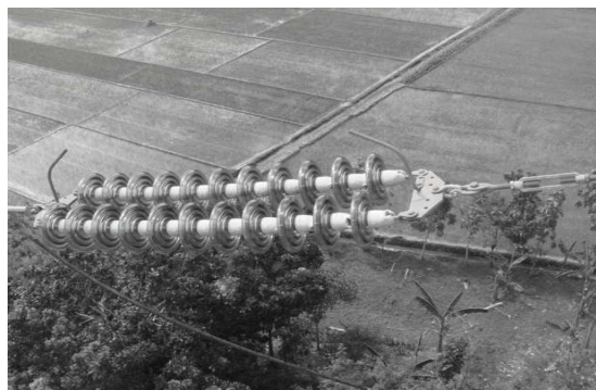
Gambar 8 Insulator horizontal string
