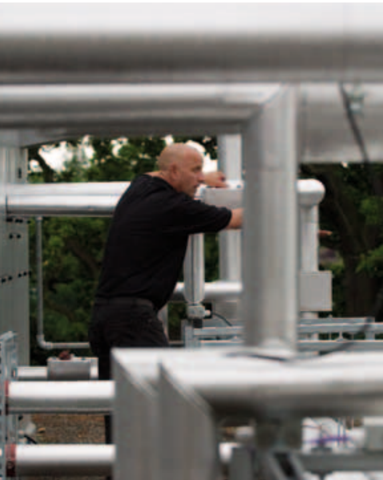
Air conditioning on the roof of Woking's leisure centre, powered by a trigeneration plant that offers cooling for extra emission savings. ©Greenpeace/Cobbing.
