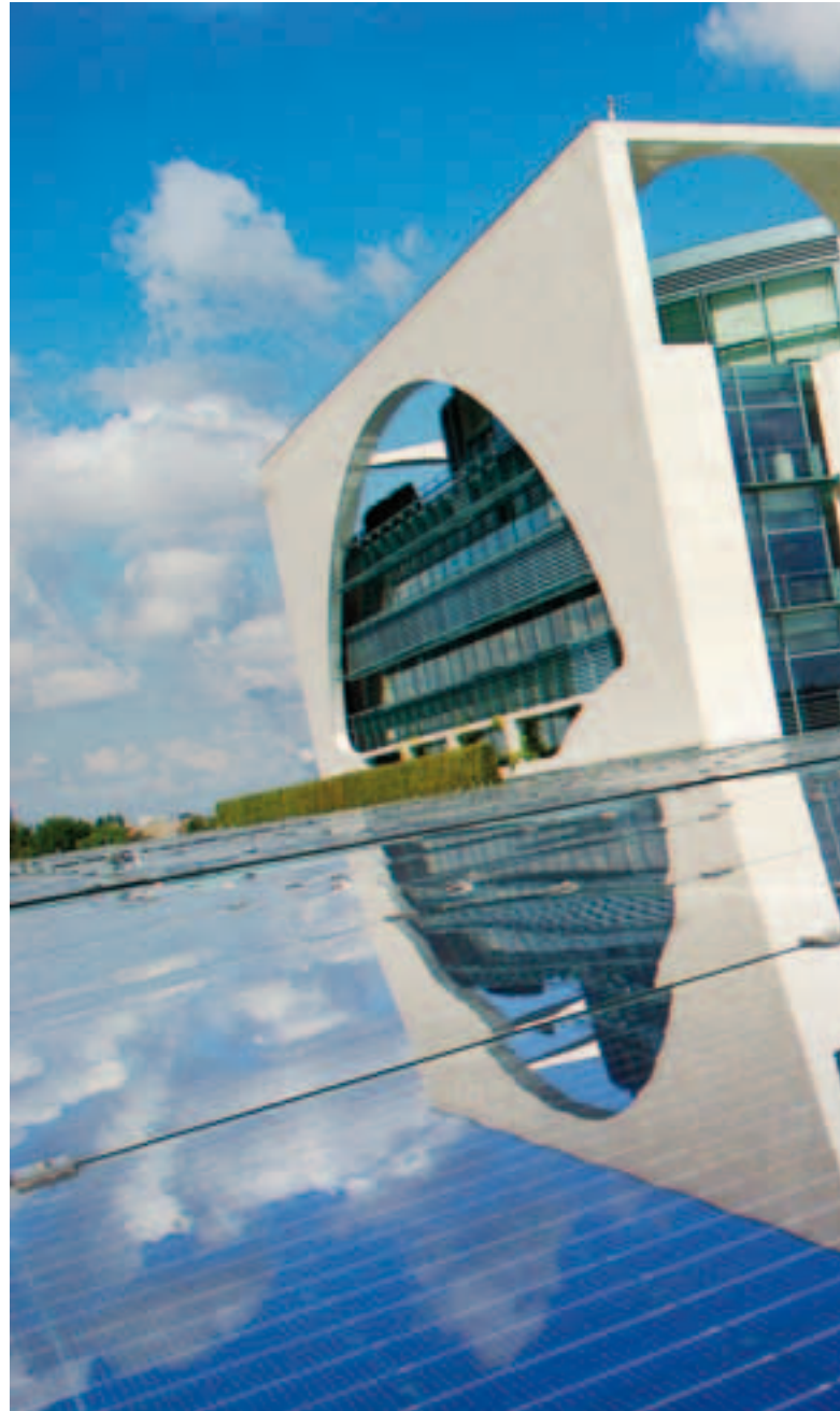
The photovoltaics facility on the roof of Berlin's Federal Chancellery shows leadership on climate change.
