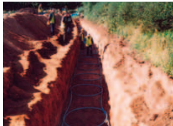
Laying a ground source heat pump means that warmth from the earth can be used to heat buildings. ©Marches Energy Agency.
