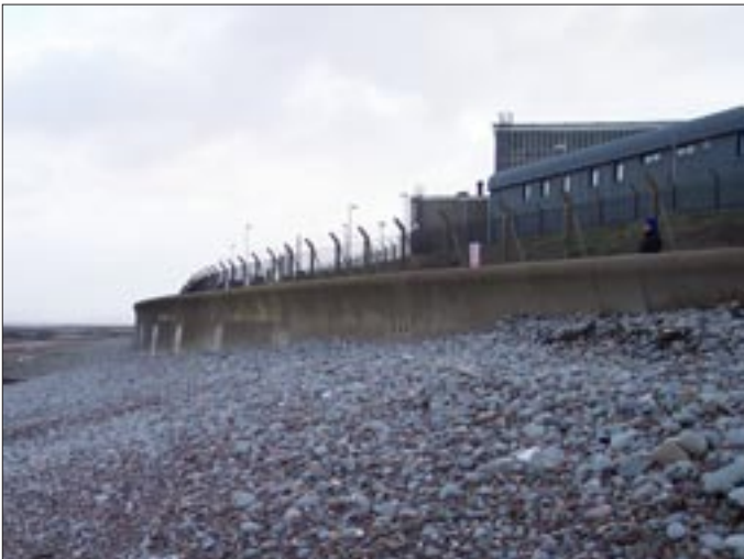
Photos 3 and 4. Extensive gabions and seawall comprise the defence structure for the power station. Increases in storm surge heights and frequency of storm events could undermine the integrity of this system and result in inundation at the site.
