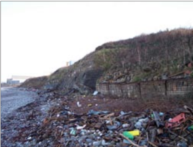
Photo 5. Additional cobble gabions protecting sections of the cliff to the west of the station.
