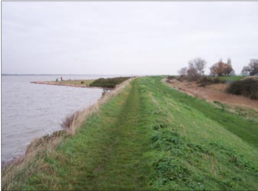
Photo 6. Considerable topographic differences either side of the embankment significantly increases the vulnerability of the power station to flooding from future climate change.
