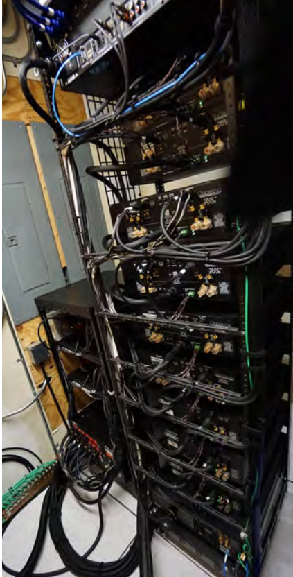
Rear of the rack shows attention to detail
