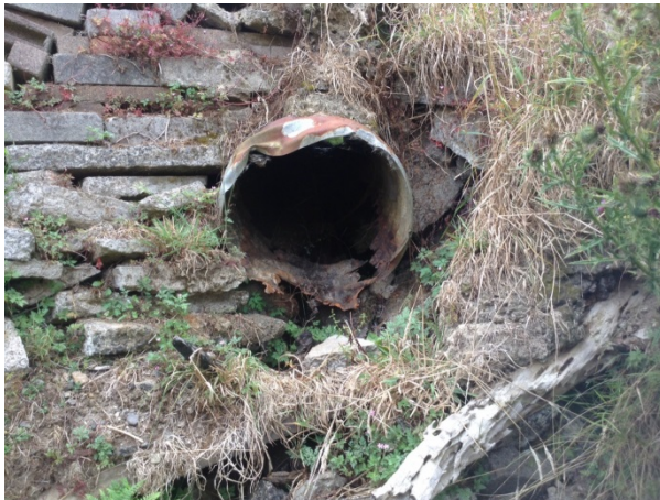
Figure 92: Culvert in poor condition upstream of MGK_E_Trib4_2.
