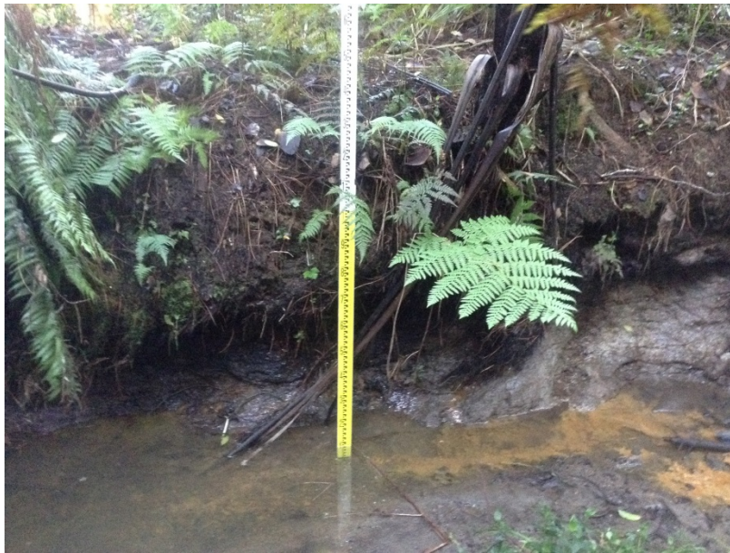
Figure 137: Bank undercutting along MGK_W_Trib1_Fork1_1.
