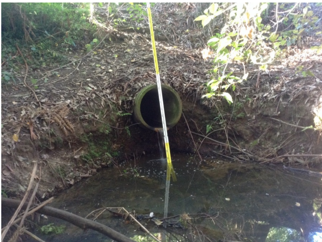
Figure 120: Perched culvert presenting a fish barrier in low flows.
