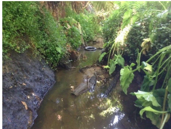
Figure 142: MGK_C_Main_2 assessed as poor land slope, poor mass wasting, poor debris jam and good vegetation. Overall stability score is poor.
