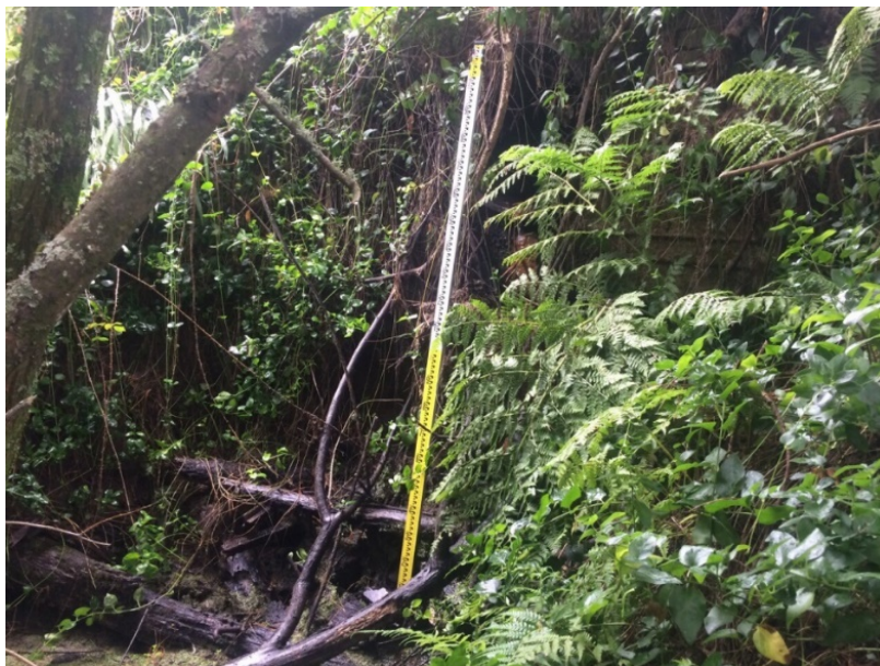
Figure 127: Fish barrier at perched culvert under farm crossing upstream of MGK_E_Trib3_3.
