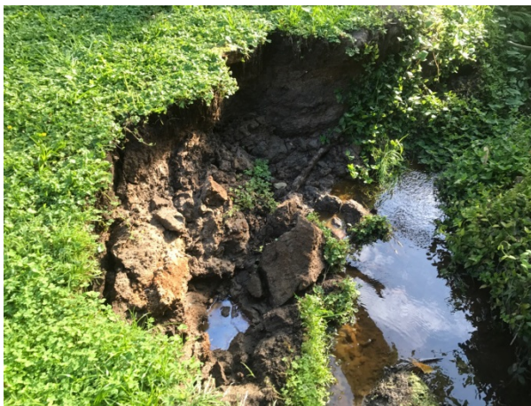
Figure 50: Erosion hotspot at MGK_W_Trib5_2.
