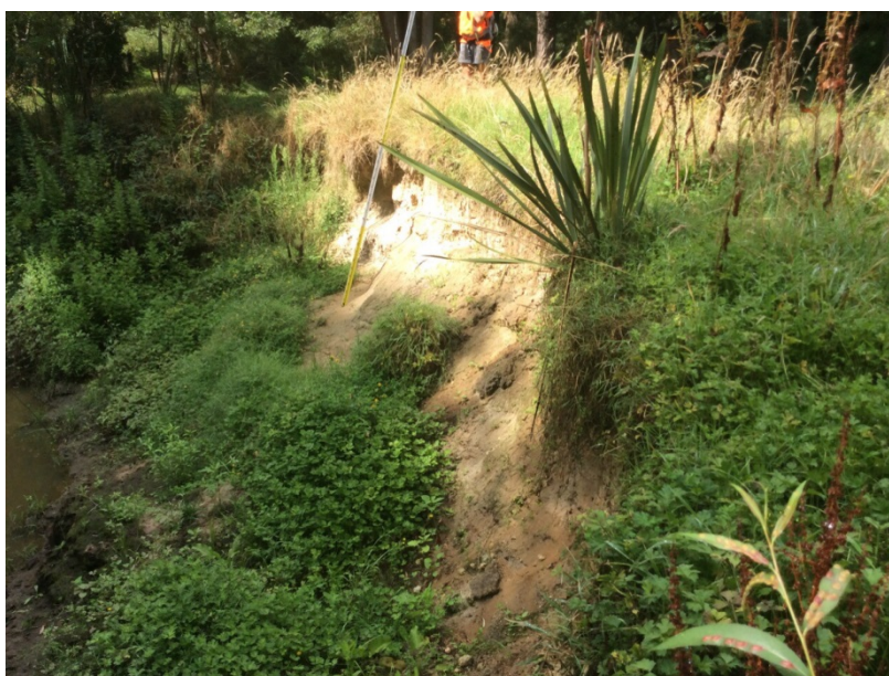
Figure 130: Erosion Hotspot along MGK_Main_2.
