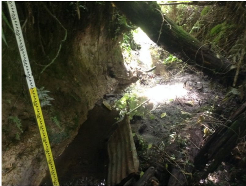
Figure 134: Erosion and scour along MGK_C_Trib2.
