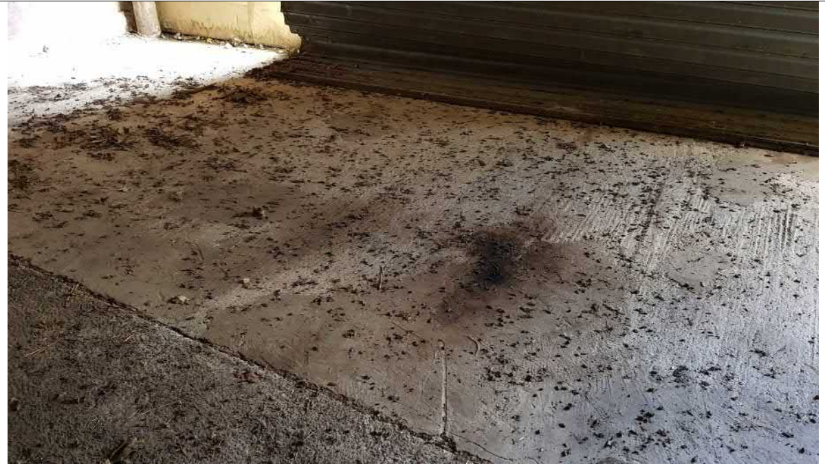
Photo 1. Hydrocarbon staining on floor of shed, facing west. Lot 5 DPS 15123.
