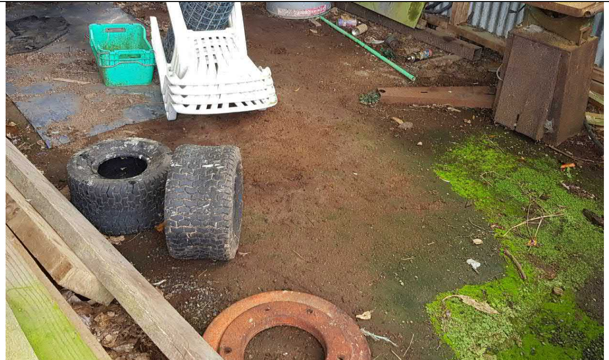
Photo 5. Potentially hydrocarbon stained soil, inside barn facing north-east. LOT 6 DPS 15123.
