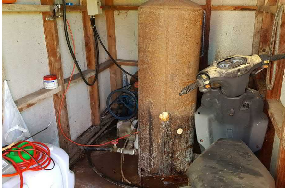
Photo 3. Unknown metal tank (leaking) with generator & herbicide tank, facing west. SEC 23 SO 495676.
