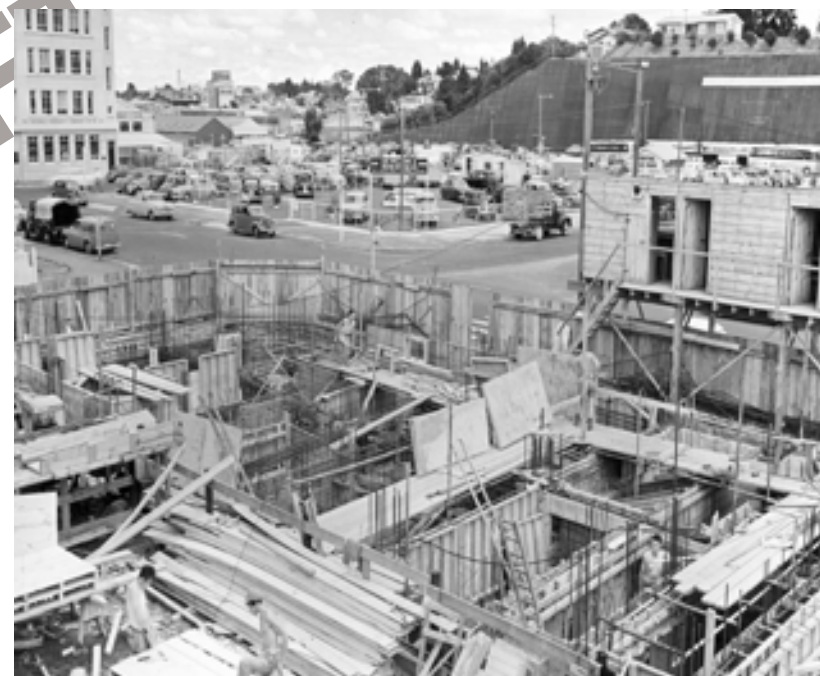
Figure 4.39 The M.L.C. building under construction in 1957; this was another of the substantial buildings in Garden Place built by Fletchers. The National Insurance building is at top left. Fletcher Trust Archives 9204P/45.
