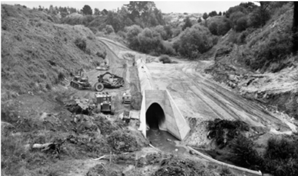
Figure 5.34. Once the concrete culvert was completed, the Waitewhiriwhiri Stream gully was in-filled. See also Figure 1.11 for a later stage in the process. Photographer: A.E. Graham. HCL_04706.
