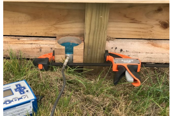
Figure 9: Vibration monitoring for structural damage. Vibration monitoring device set up on a building pile using a piece of wood clamped to the pile. The transducer sits within the block of wood.
