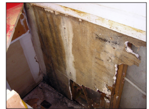
A slow leak caused mold to grow behind this counter. After a plumber fixed the leaky pipes, we came to remediate the mold.
