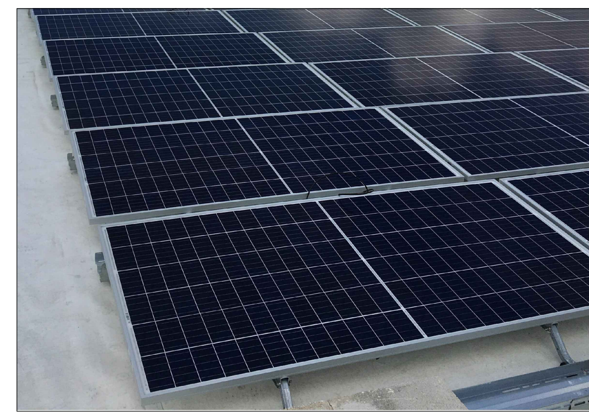
TYPICAL PANEL CLAW RACKING ARRANGEMENT
