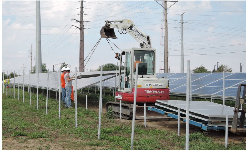
The University of Illinois at Urbana-Champaign's strategic planning efforts have resulted in aggressive energy goals. A new 20.8-acre solar farm is currently under development. Photo credit: Tony Mancuso, Institute for Sustainability, Energy, and Environment.
