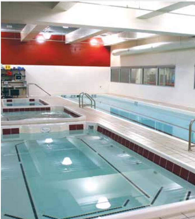
The hot and cold plunge tanks in the Holthus Family Hydrotherapy area help the Huskers recover after workouts and injuries.
