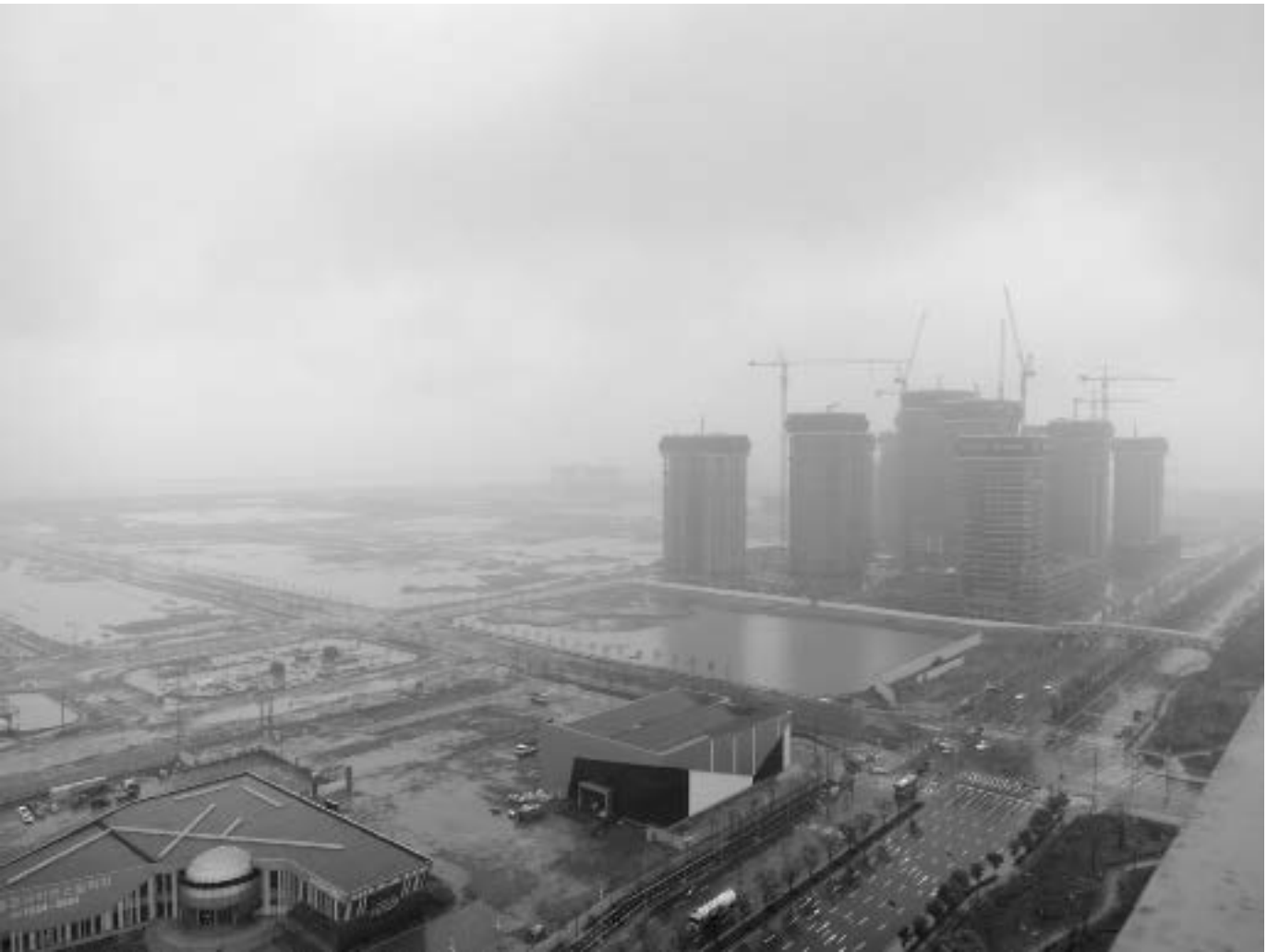
Figure 1 Songdo International Business District under construction, Incheon Free Economic Zone, South Korea, July 6, 2012. (Image: Jesse LeCavalier)
