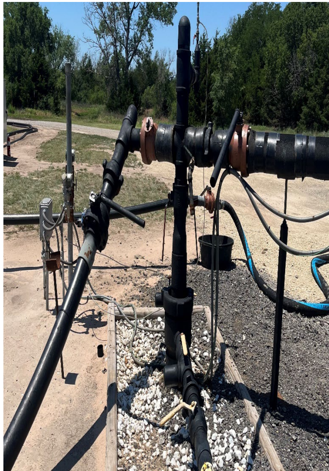
Figure A3-3. SW-12 Wellhead manifold.
