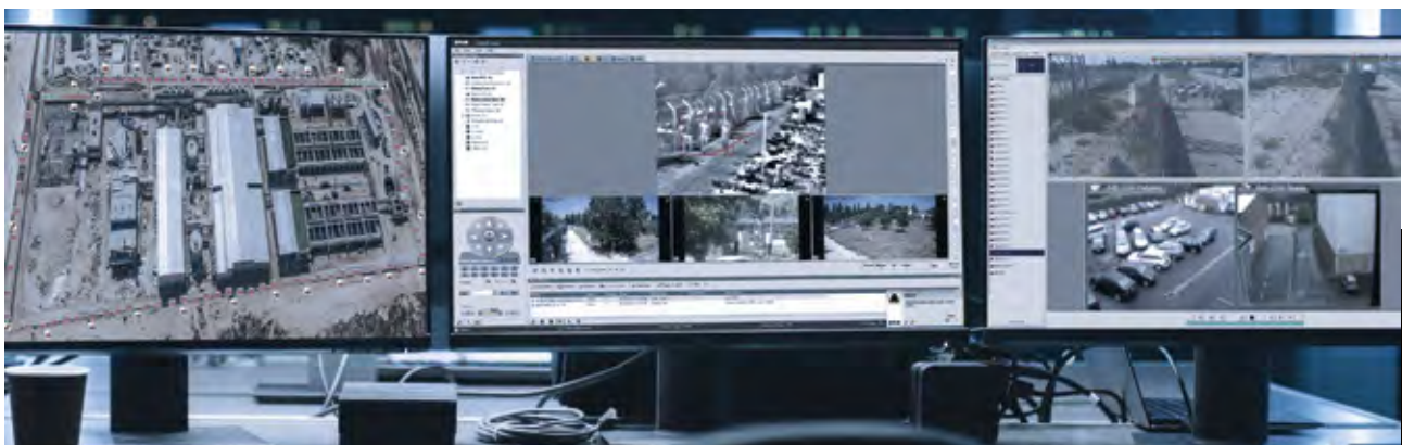
Integrated Video Surveillance & Smart Fence Operation Display
