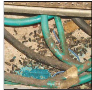
Rat droppings at the bottom of an electrical cabinet
