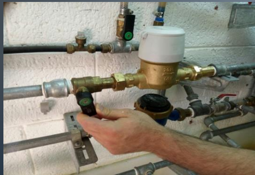
Turn on the water flow stream
