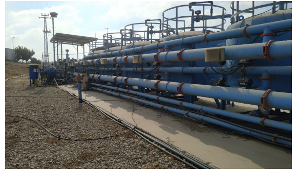
Effluent Tertiary Treatment plant- General view
