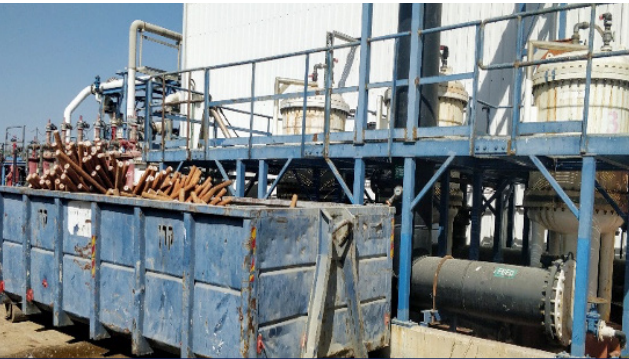
Maagan Desalination is the largest Brackish water desalination plant in Israel. Almost 1000 cartridges are dumped every time.
