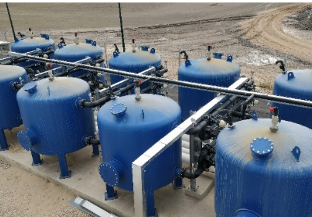
The array of Sand filters in Afkey Mayaim Desalination plant
