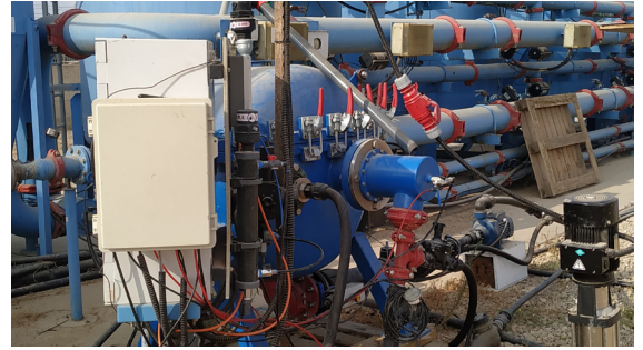
Fiber Disc Filter pilot unit- General view
