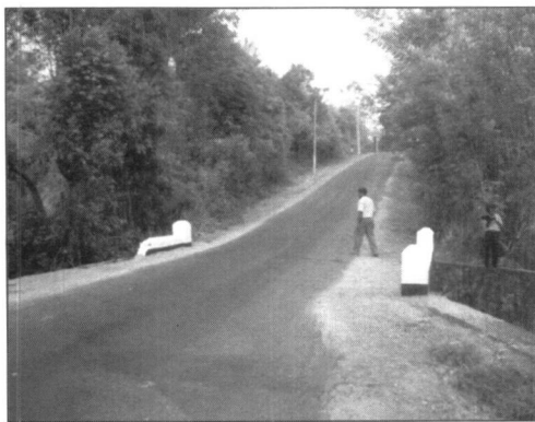
Figure 7: A View of the case study bridge (bridge Number 43/2) in B312 route
