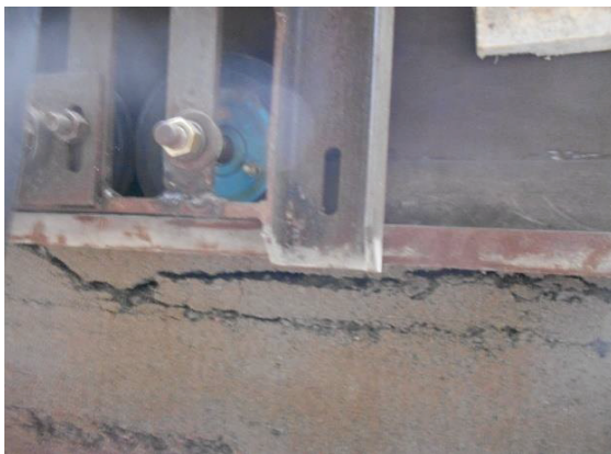
Figure 18 - Horizontal Cracks Propagate During Shutter Lifting
