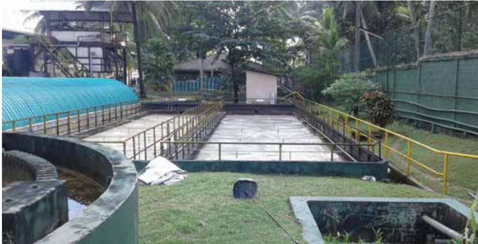
Figure 3: A Water Treatment Plant of a Soft Drink Manufacturer
