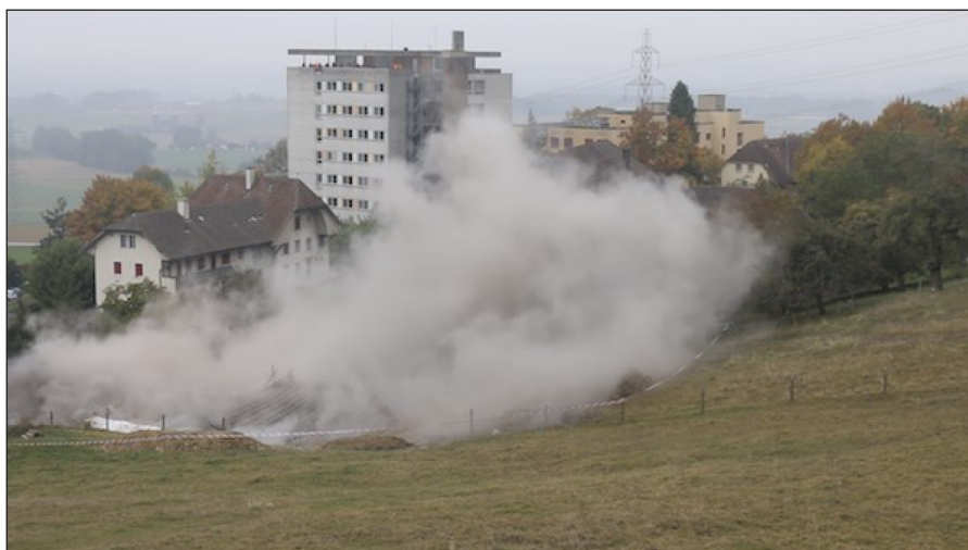
Still image from the filmic research journal. Explosion of an old building on the site of a future Alzheimer care "village".
