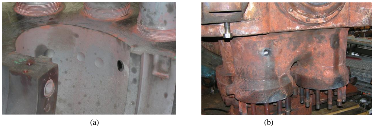
Figure 3. (a) Sampling marks on the inner surface of bottom part of turbine case body GT201, (b) Sampling marks on the outer surface of upper part of turbine case body GT201.
