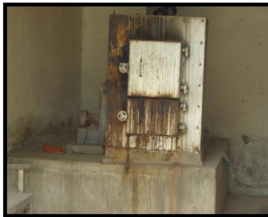
Figure No 9: Showing Incinerator which is not in working condition
