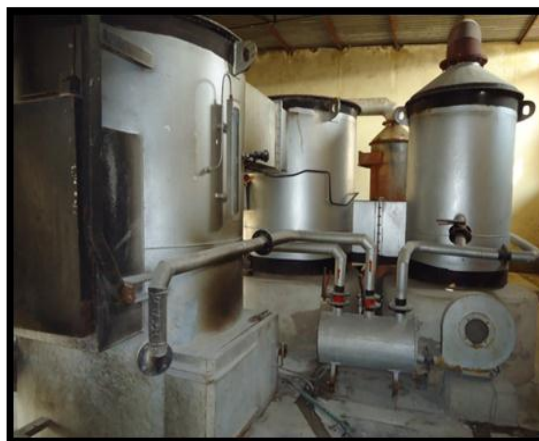
Figure No 11: Showing incinerator at CBMWTF of Ajmer
