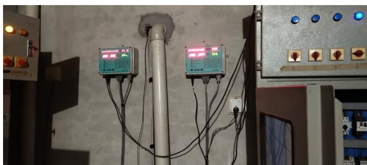
Figure 01: Continuous power supply with temperature check.
