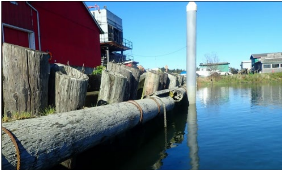
Figure 3: Damaged East Bulkhead Wall (GeoEngineers Report)
