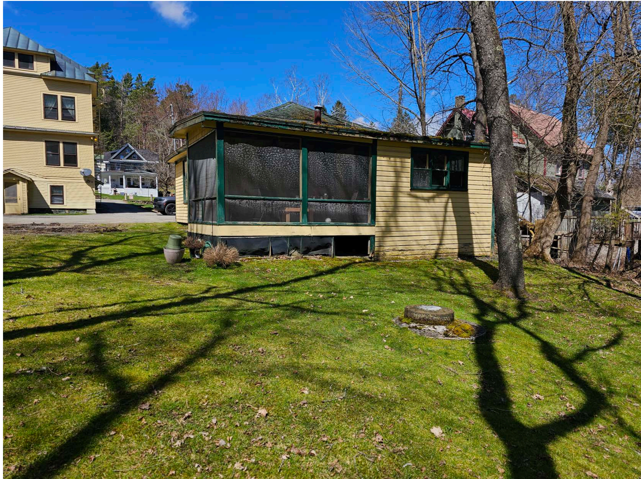
REAR VIEW OF EXISTING TWO (2) BAY GARAGE TO BE REMOVED FOR NEW BUILDING 2 (LOCATED INSIDE TOWN OF ST. ARMAND, ESSEX COUNTY) EXISTING SEWER MAIN LOCATION SHOWN
