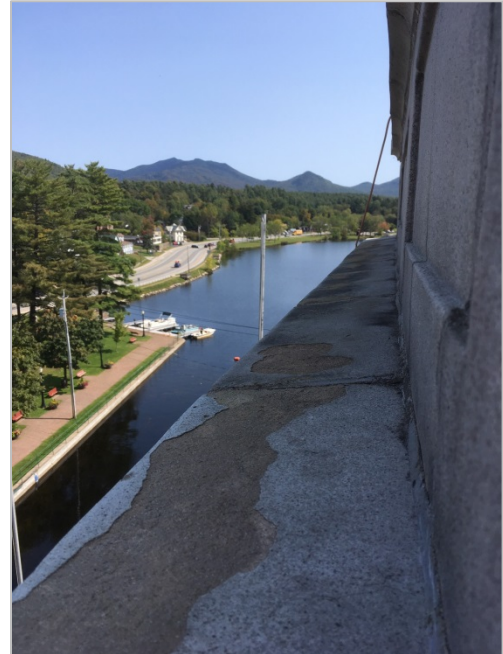
Typical terra cotta glaze damage on horiz. ledge.
