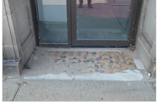
Damaged original glazed tile & marble entry floor
