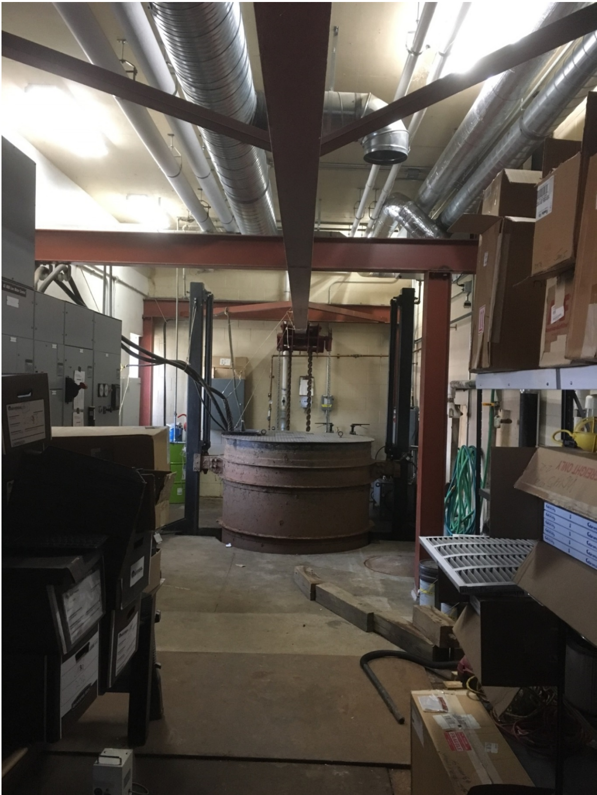
Interior of Hydro-Electric Plant – looking east
