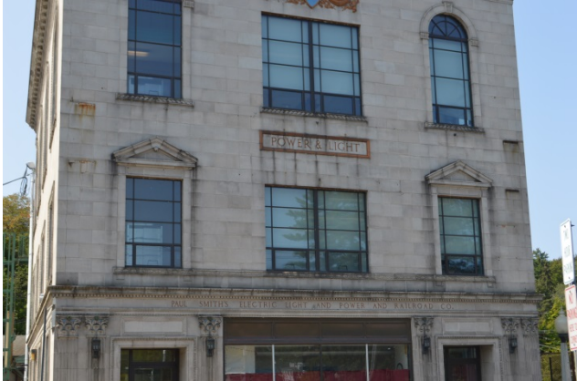
East elevation showing rust staining from iron fasteners
