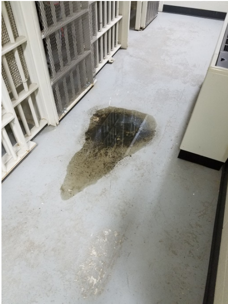
Jail Cell area – sewer backflow
