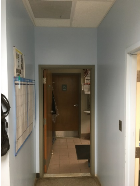
Corridor to Staff Toilets–narrow clearance
