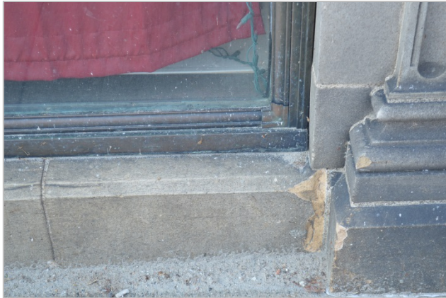
Evidence of freeze-thaw damage along Main St. sidewalk
