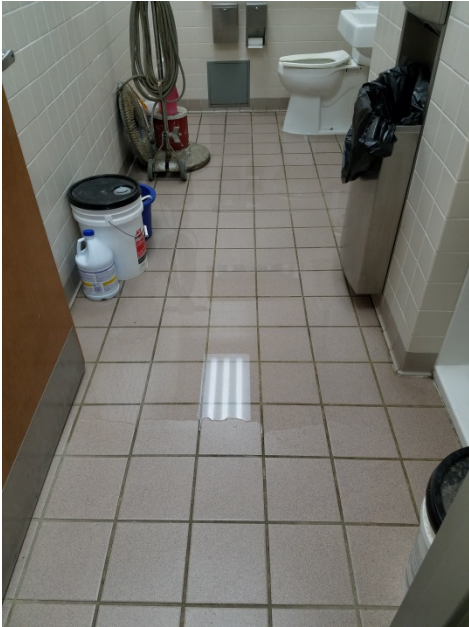
Staff Women's Toilet – sewer backflow
