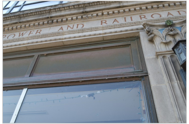
Original storefront & transom window—missing glazing
