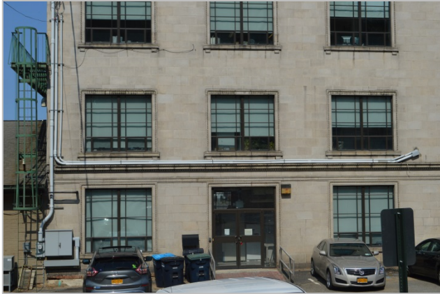
South elevation with modern, visually obtrusive utilities.
