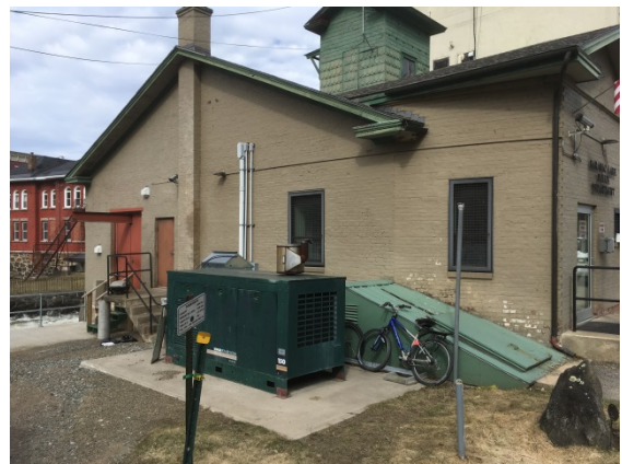
Generator and basement access doors along west side.
