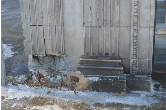
Impact damage of terra cotta base at SE corner
