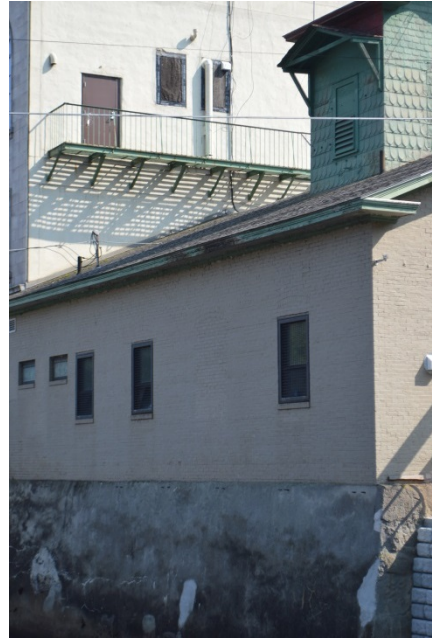
North roof eave exhibiting paint failure
