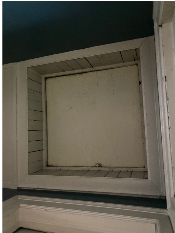
Roof hatch framed with beaded boards walls located in ceiling of short hallway.
