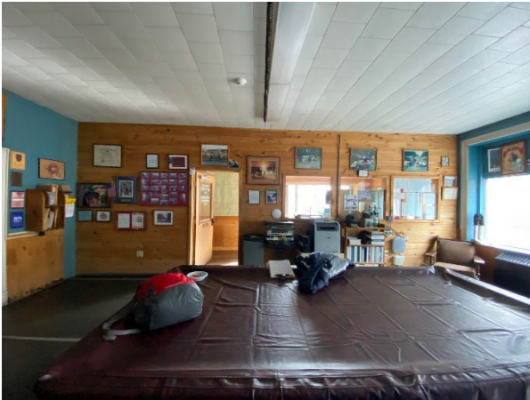
Modern south partition wall of Day Room constructed of knotty pine boards & fixed windows – out of character of orig. finishes.
