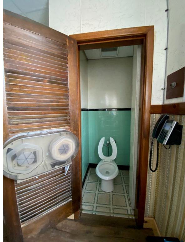
Mid/late 20 th century fixtures and finishes are showing age and wear.
