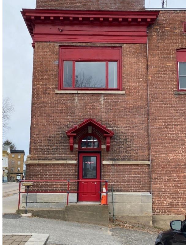
Original side entry with replacement door and framed down and altered 2 nd floor window.
