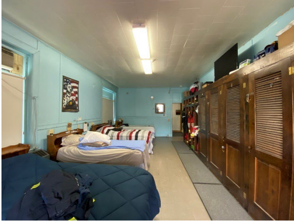
Historic wall, ceiling and floor finishes covered with layers of vinyl tile, acoustical tile and Masonite sheet paneling.
