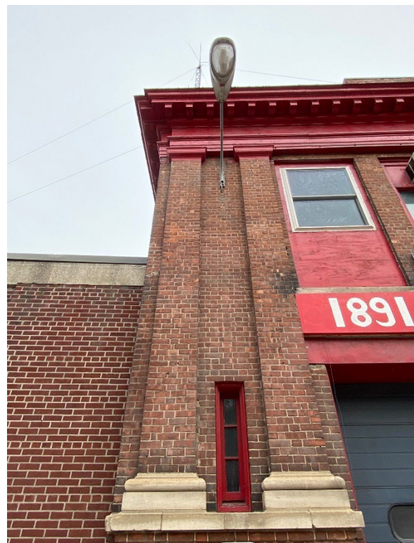
Pressed metal entablature/cornice painted red. Note stone pilaster capitals also painted red.
