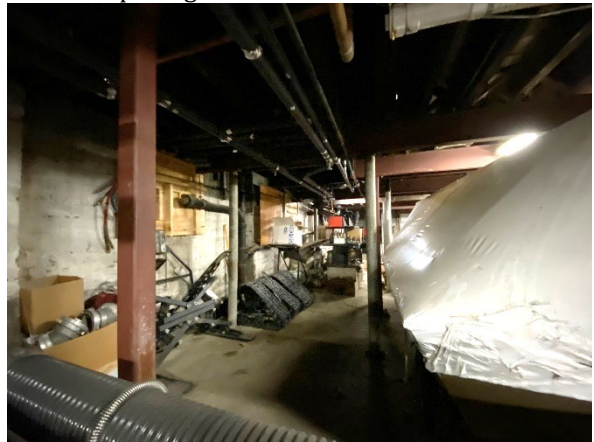
View of parge-d foundation wall on north side of basement with former window openings to crawl space of 1960s addition infilled with plywood.
