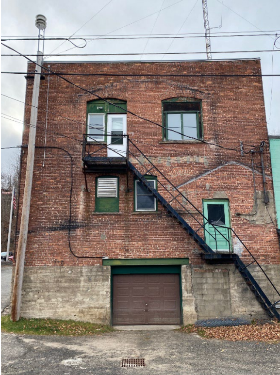
Rear east elevation with ghost lines of former 2 nd floor bay window and gabled roof of NE addition.
