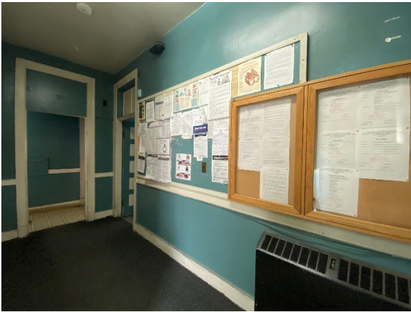
2 nd floor stair hall with original trim elements intact on 3 of 4 walls. Note tall doorways with transoms.
