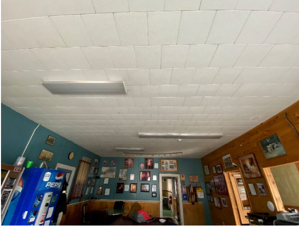
Interlocking acoustical ceiling tiles within Day Room with surface mounted fluorescent lighting.
