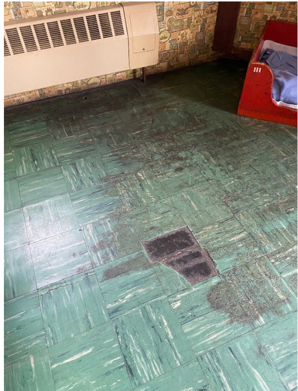
Vinyl composition tile (VCT) on floor is in poor condition in many locations. 9" square VCT typically contained asbestos & is considered a HAZMAT.
