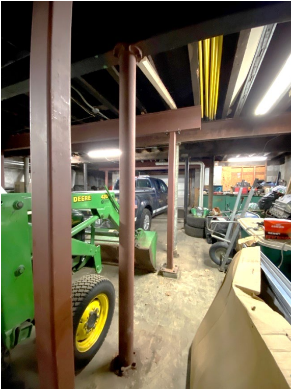
View of row of metal columns in random positions to support added steel beams for first floor framing.
