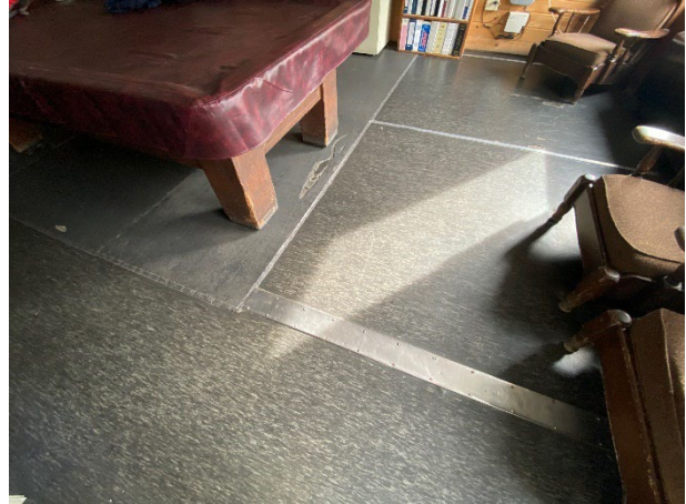
Linoleum sheet flooring pieced together with stainless steel threshold strips. Likely over orig. wood flooring.
