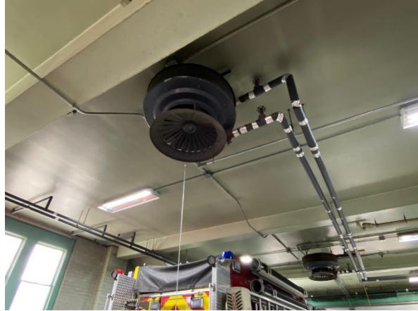
Note exposed electric, piping and equipment attached to ceiling.
