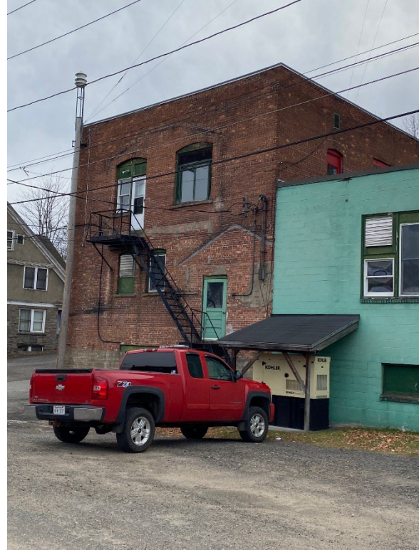
View of north elevation showing altered window openings and c.1960s CMU addition.
