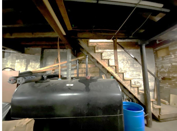
Looking south at staircase along parge-d foundation wall. Note oil tanks with filler pipes through former window opening.
