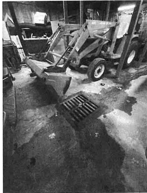
Large drainage grate positioned in center of basement floor for site water from rear yard.
