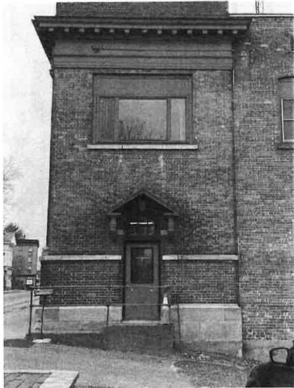
Original side entry with replacement door and framed down and altered 2 nd floor window.
