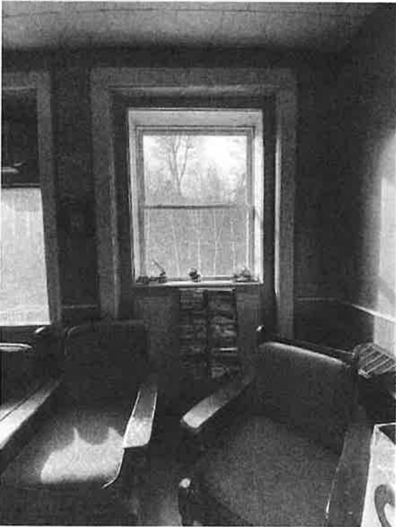
Detail view of orig. doorway opening to front balcony, now infilled with a small window unit.
