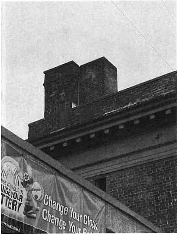
Metal entablature returned on north elevation. Note brick parapet & orig. chimney with new boiler chimney added next to it.
