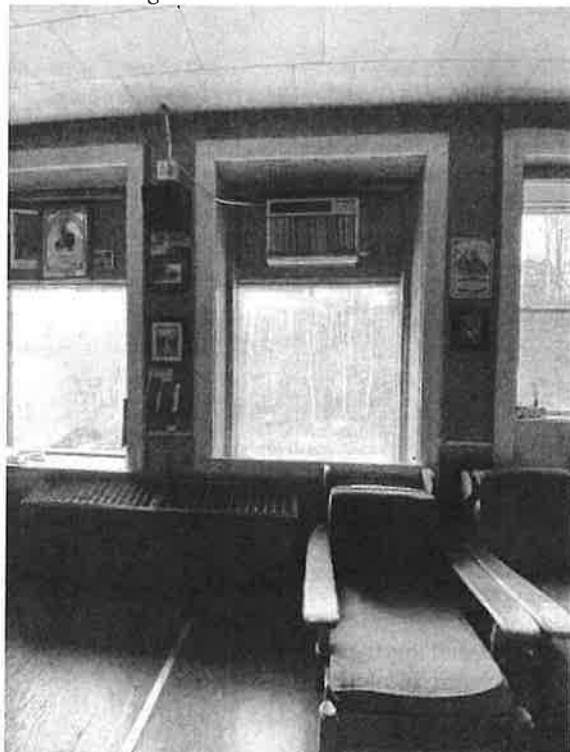
View of centered windows on front wall of Day Room with plywood infills and fixed window units replacing orig. double hung sash.
