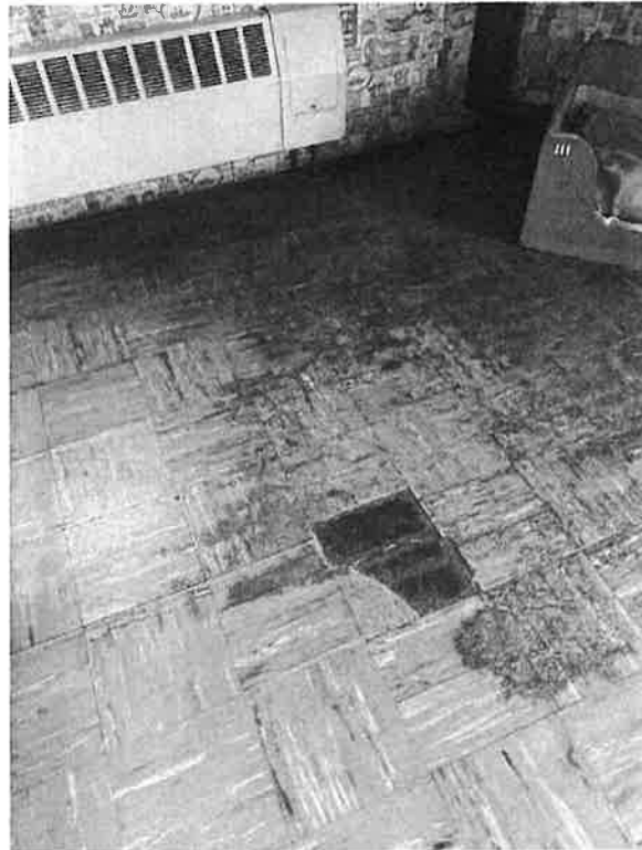
Vinyl composition tile (VCT) on floor is in poor condition in many locations. 9" square VCT typically contained asbestos & is considered a HAZMAT.
