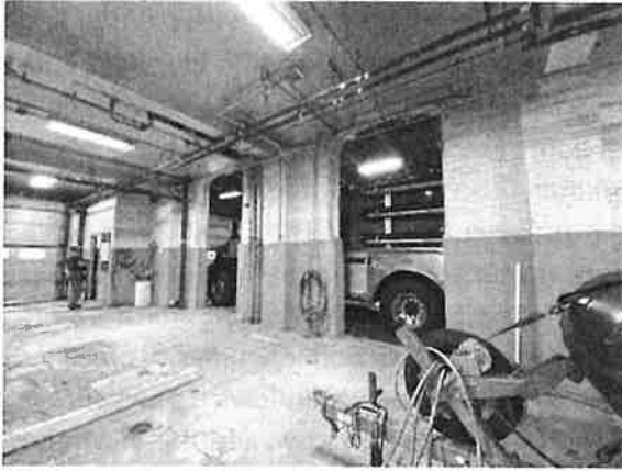
North wall where orig. window openings have been opened to created doorways to new addition.
