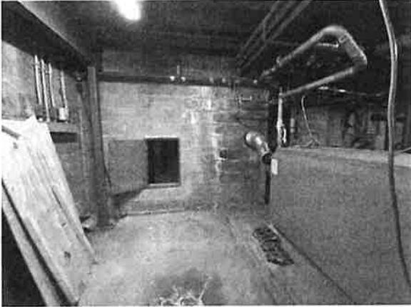
View of wall of hose tower with access door. Note new boiler exhausts into new chimney built within hose tower.
