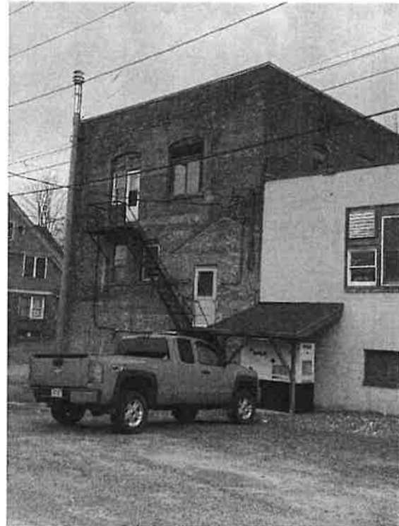
View of north elevation showing altered window openings and c.1960s CMU addition.
