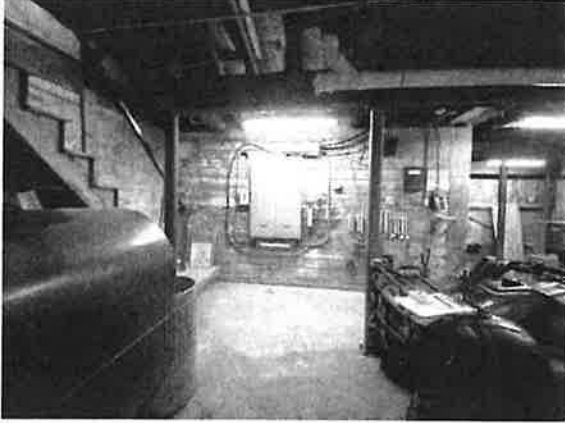
Shiplap board partition wall at bottom of stairs in SW corner – former coal bin. Note new elect. panel.
