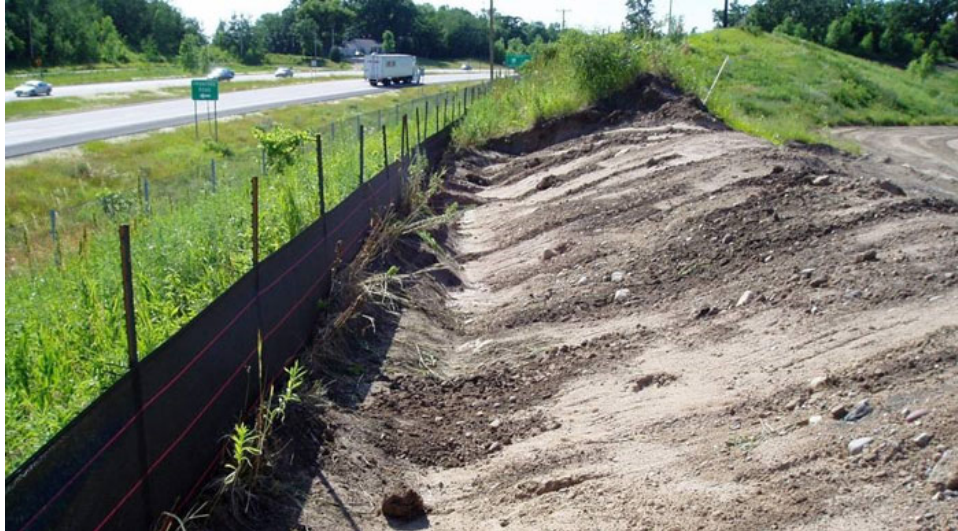
Figure 8: Installed silt fence will minimize sediment leaving a site and contaminating surface waters
