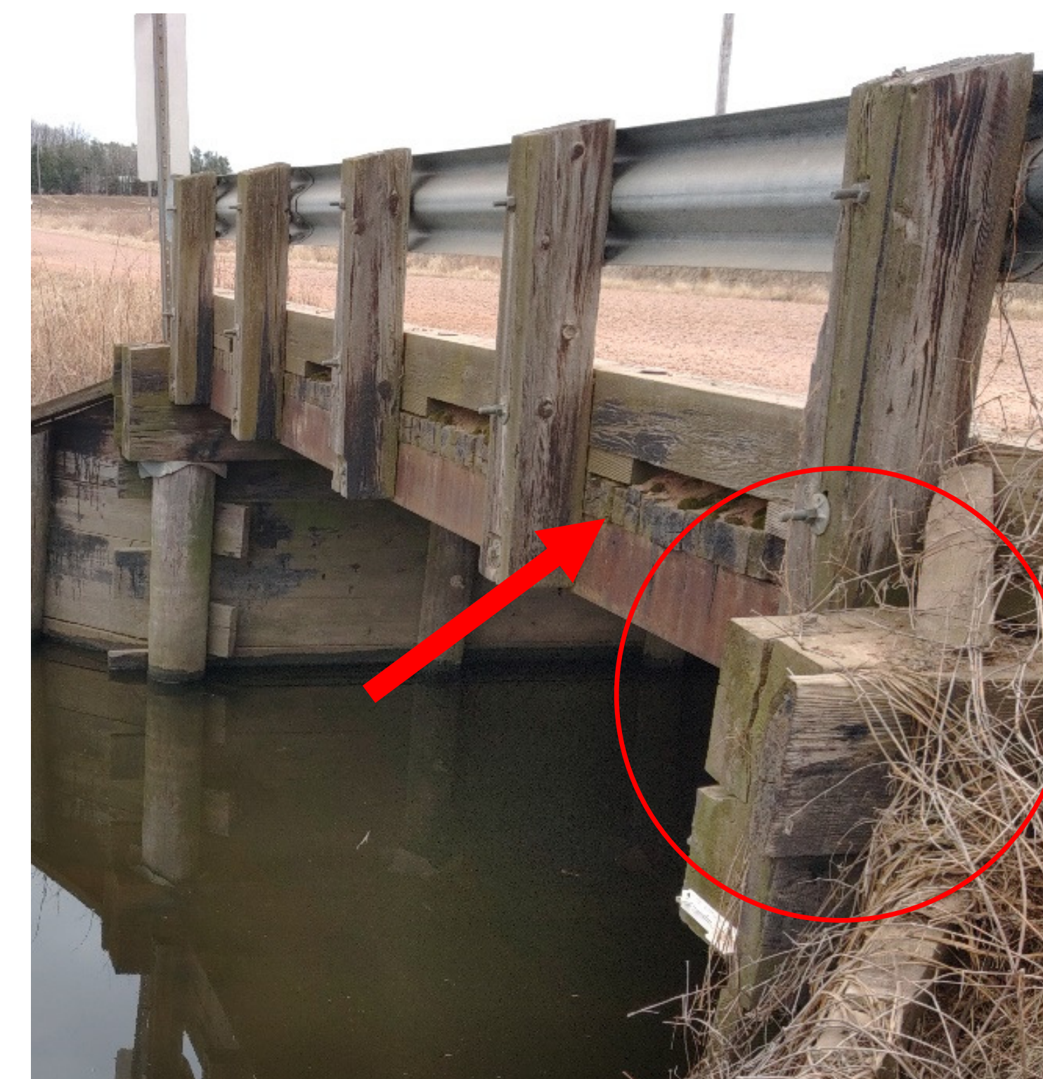
Figure 2: Deteriorating timber deck evident (arrow) as well as cracked timber cap (circle).
