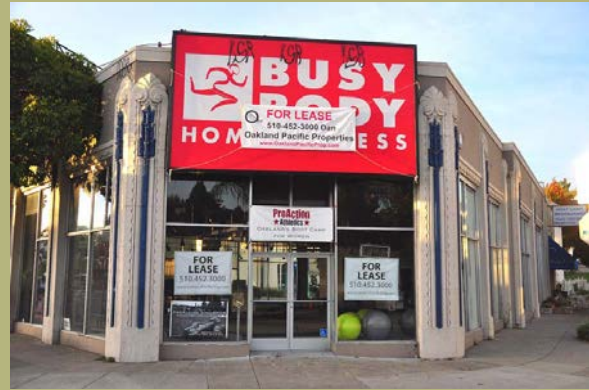
NOT PERMITTED This wall sign obscures the existing architectural features, including part of the windows, and is out of proportion to the building mass.
