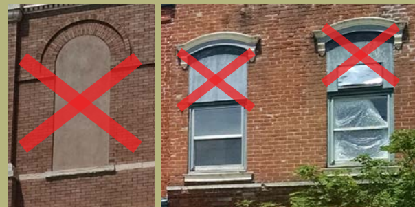
NOT RECOMMENDED Filling of window openings with wood, brick, or any other materials is discouraged.
