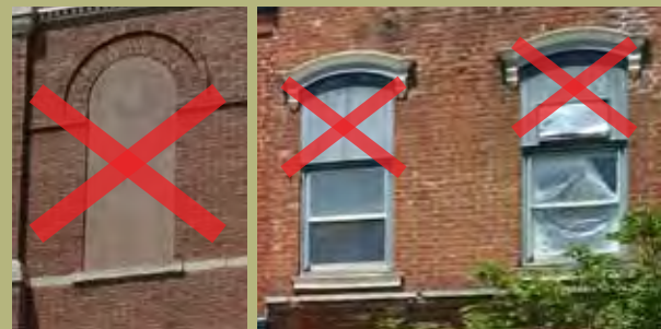
NOT RECOMMENDED Filling of window openings with wood, brick, or any other materials is discouraged.
