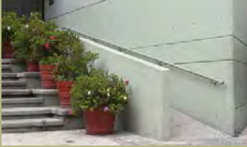
APPROPRIATE The ADA ramp is incorporated in the stair entrance and meets the needs of all users.
