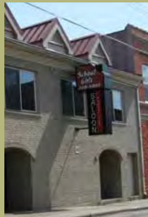
NOT PERMITTED The projecting sign is placed in front of a window while an alternative location between the windows is available.
