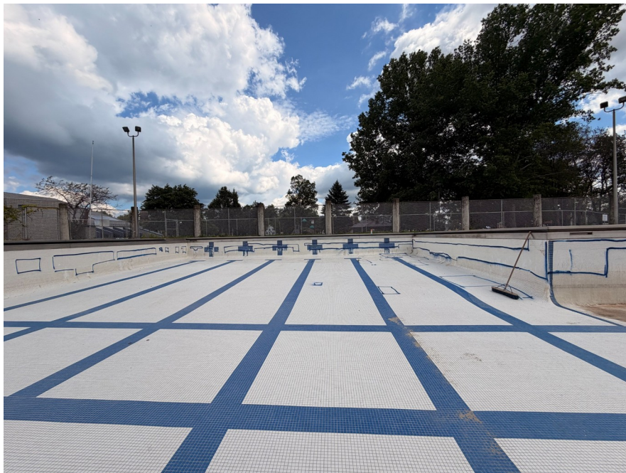
Photo 2 Opposing overview of the pool. Marked wall areas and localized floor areas are visible within the existing tiled finishes.
