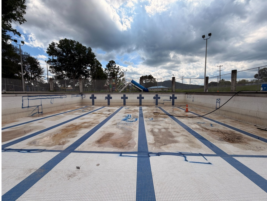
Photo 1 View toward the deeper portion of the pool. Blue-painted outlines identify areas with differing sound responses on the walls and floor.
