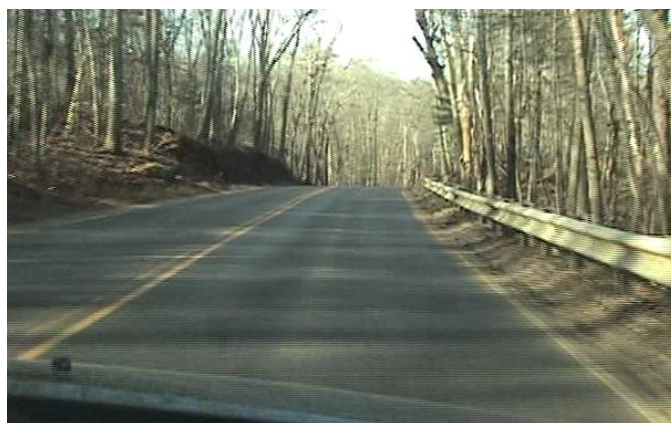
Edge Lines obstructed by sand
