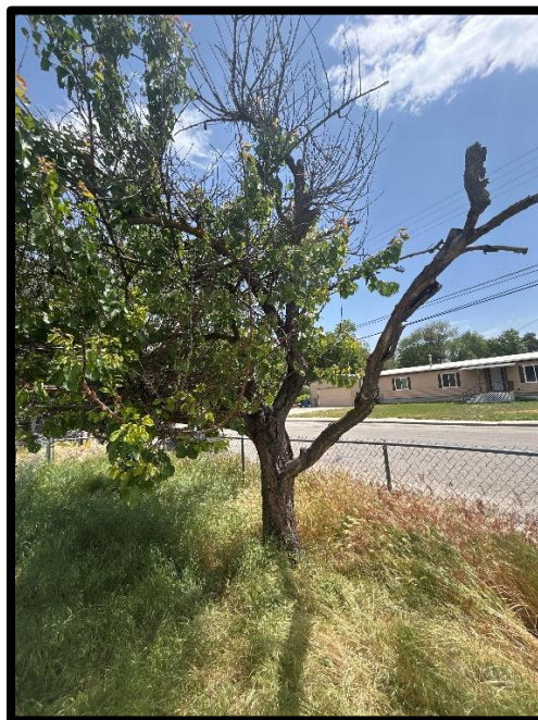
Photo 1. View of tree #1 with large areas of decay and dead.
