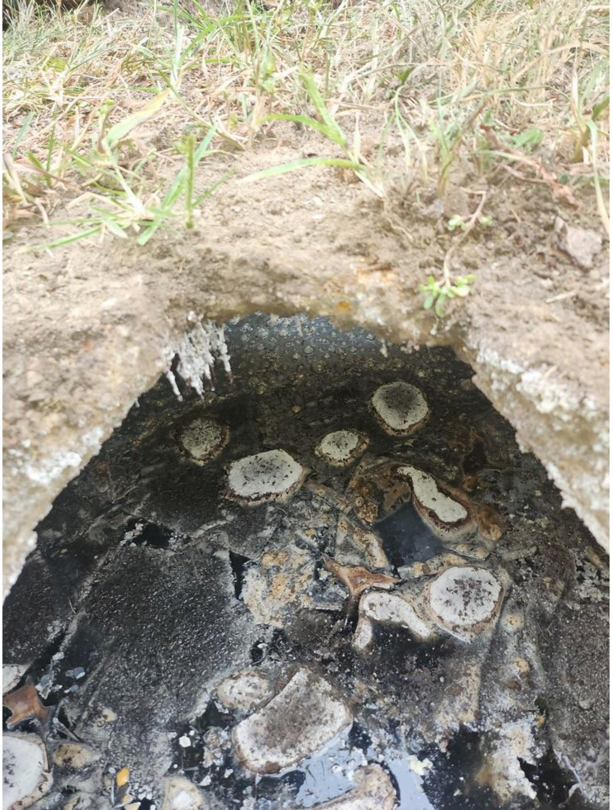
FIG. 8 - 11 FOURTH ST. FAILING SEPTIC TANK (from Morris Cooper)
