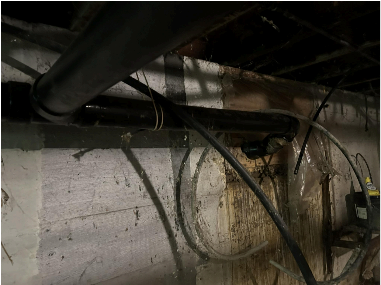
FIG. 3 - DRAIN PIPE COLLECTS OUTPUT FROM SUMP PUMPS AND DRAINS TO SEPTIC TANK (11 FOURTH ST.)
