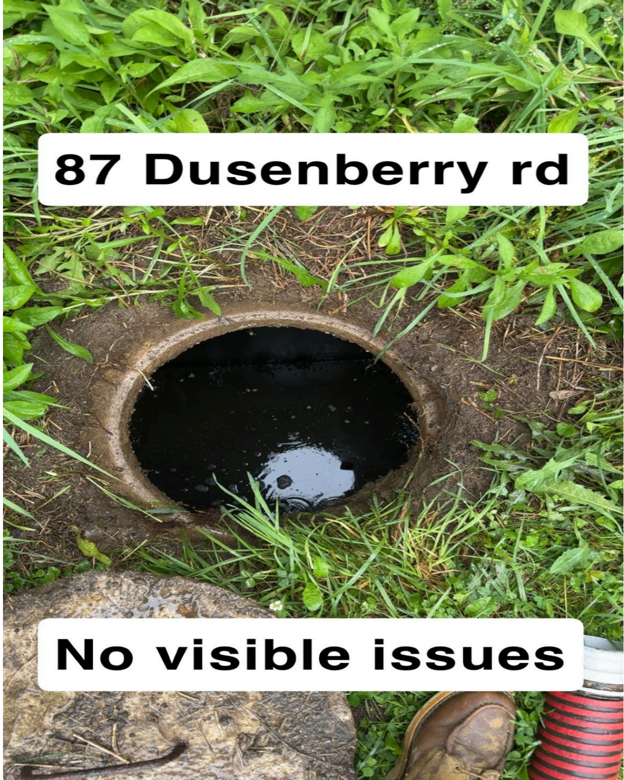
FIG. 5 - 87 DUSINBERRE RD. SEPTIC TANK
