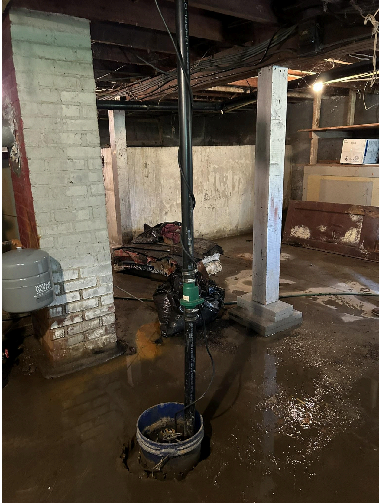
FIG. 1 - SUMP PUMP 1 AT 11 FOURTH ST.
