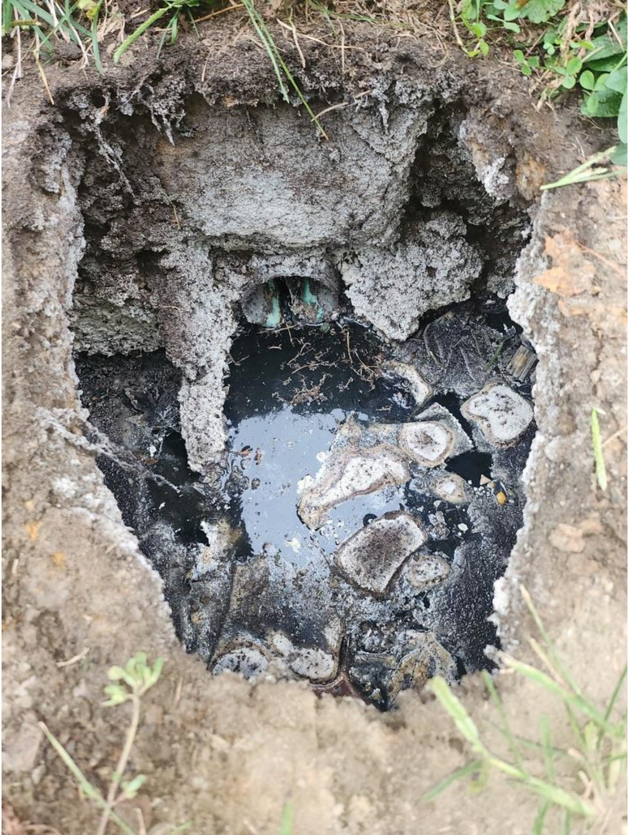
FIG. 7 - 11 FOURTH ST. FAILING SEPTIC TANK (from Morris Cooper)
