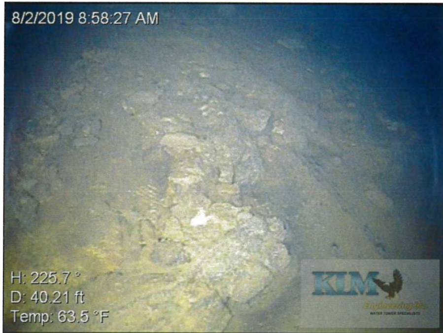
Photo No. 17 Heavy sediment accumulation and scale deposits in bowl
