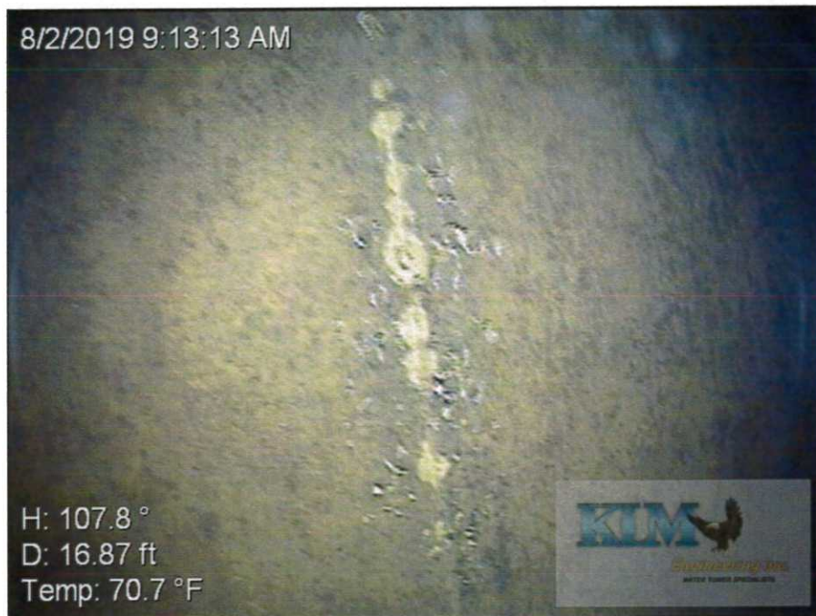
Photo No. 12 Condition of interior wet coating on shell wall Heavy scale and staining visible; coating blistering and pinhole corrosion along welds
