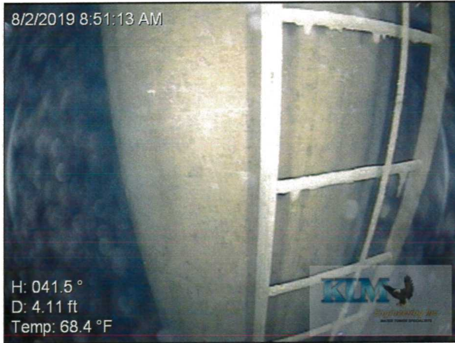
Photo No. 7 Condition of interior wet coating on drywell tube below HWL
