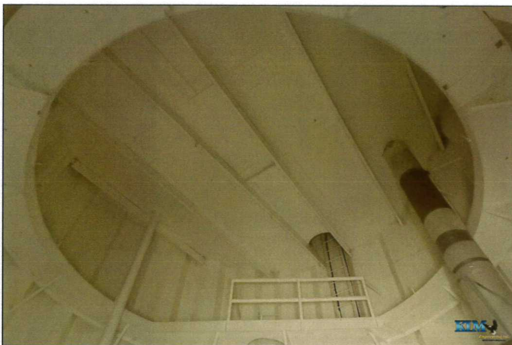
Photo No. 46 Condition of interior dry coating on bottom of condensate platform
