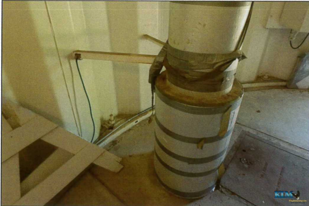
Photo No. 45 Condition of insulation and wrap on fill pipe at base of pedestal Hatch to valve pit visible
