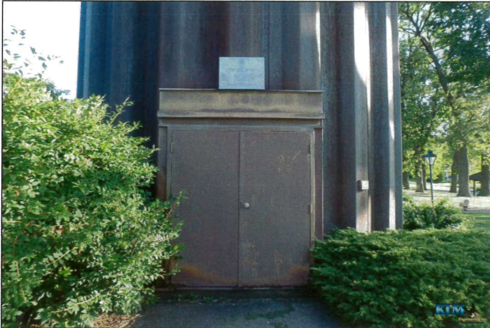
Photo No. 61 Condition of uncoated COR-TEN steel pedestal at base Double access doors significantly corroded at bottom corners
