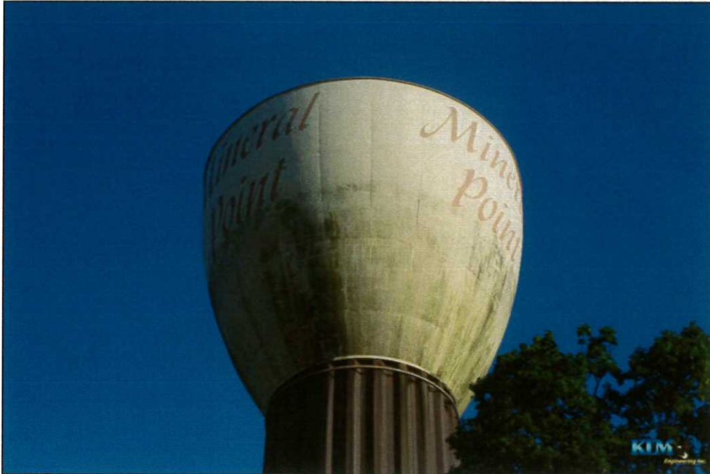
Photo No. 57 Overall condition of exterior coating on side of tank Heavy organic growth on lower half of tank
