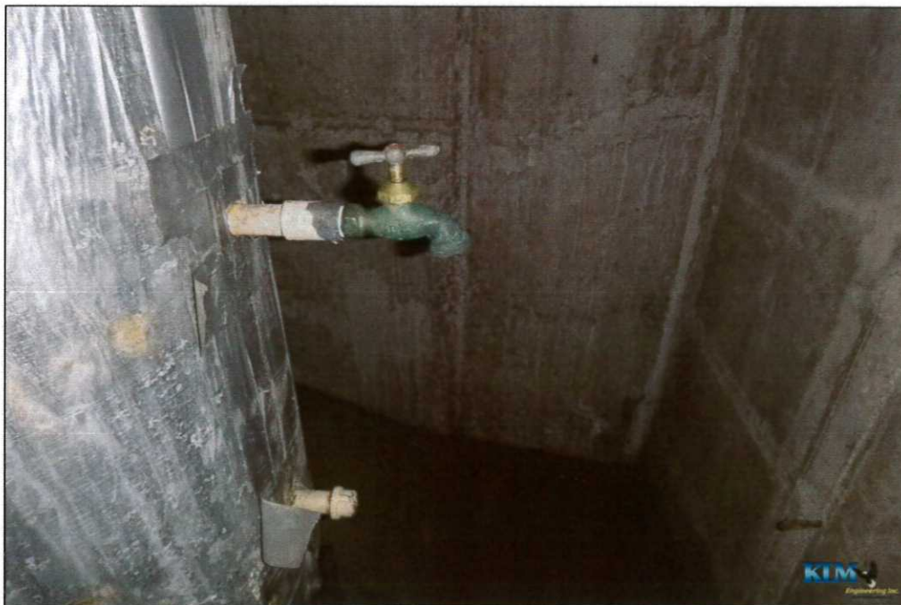
Photo No. 50 Sample tap located in valve pit
