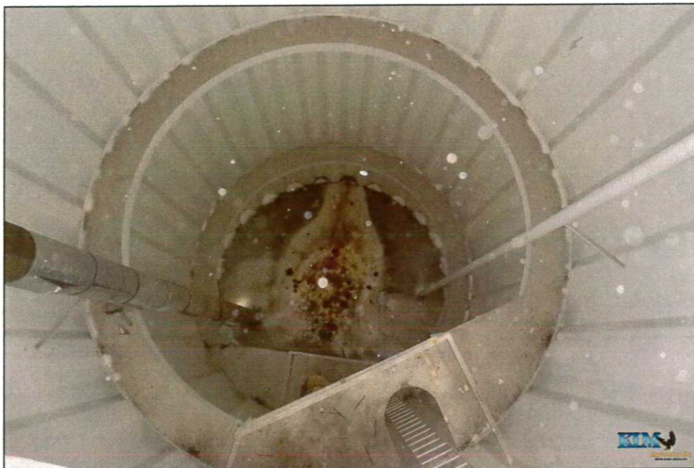
Photo No. 39 Condition of interior dry coating inside pedestal View looking down pedestal to condensate ceiling below
