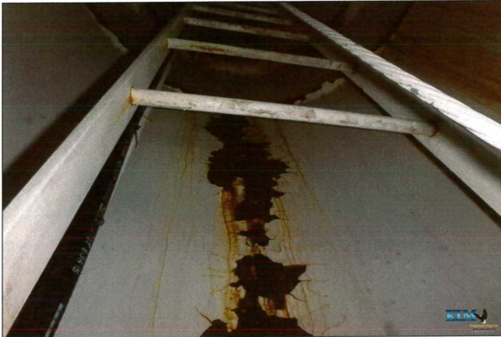
Photo No. 27 Condition of interior dry coating inside drywell tube Significant coating peeling and surface corrosion
