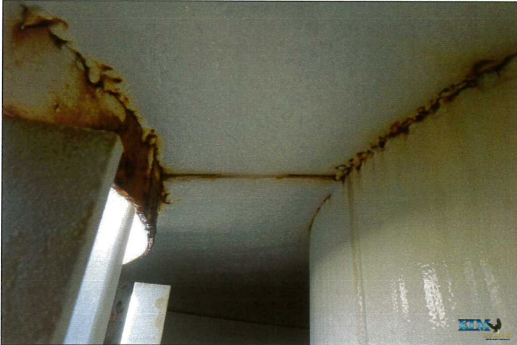
Photo No. 5 Condition of interior wet coating around drywell tube and manway access
