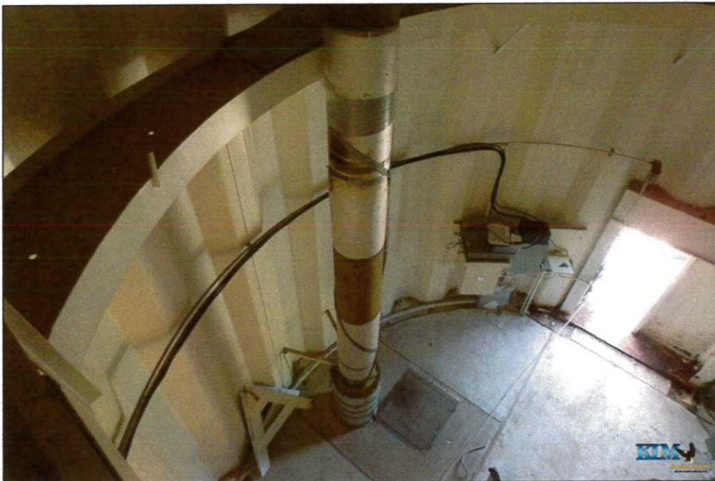
Photo No. 44 Condition of pedestal interior at base Some missing foil wrap visible
