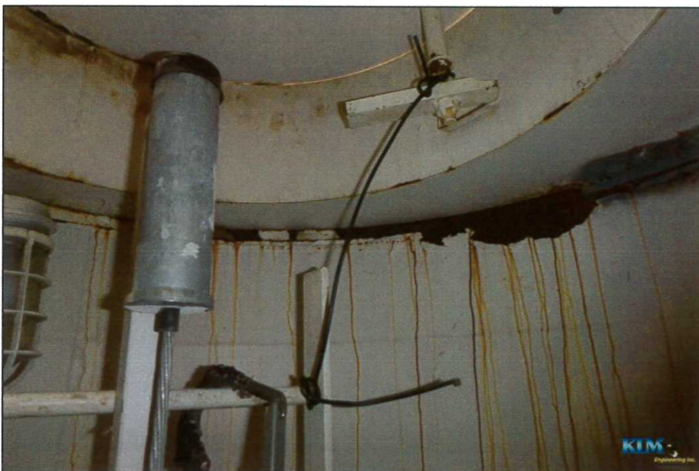
Photo No. 22 Condition of interior dry coating at top of drywell tube Significant peeling and surface corrosion occurring
