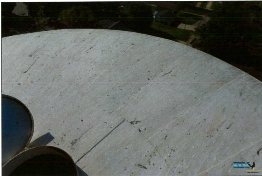
Photo No. 56 Condition of exterior coating on roof Bird droppings covering roof
