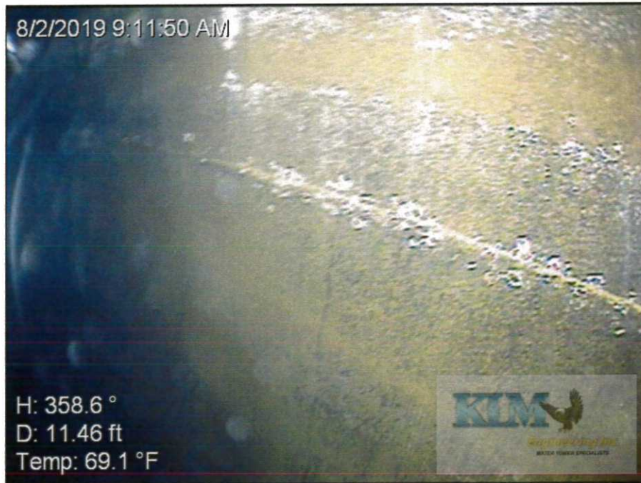
Photo No. 11 Condition of interior wet coating on shell wall Heavy scale and staining visible; coating blistering and pinhole corrosion along welds
