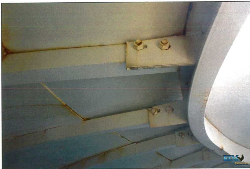
Photo No. 4 Condition of bolted rafter connections on compression ring
