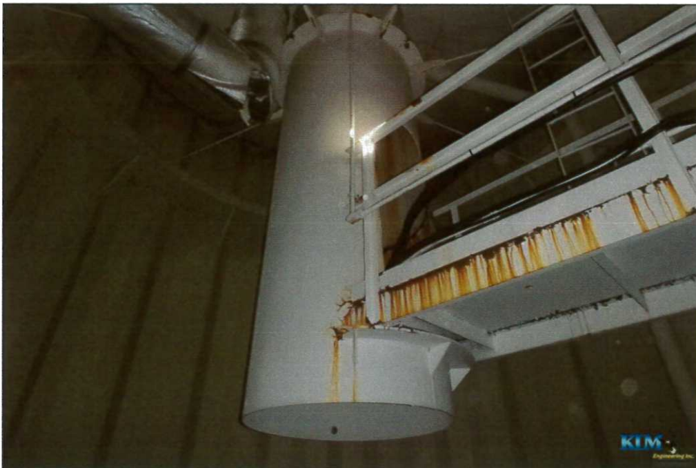
Photo No. 38 Condition of interior dry coating on drywell tube and platform
