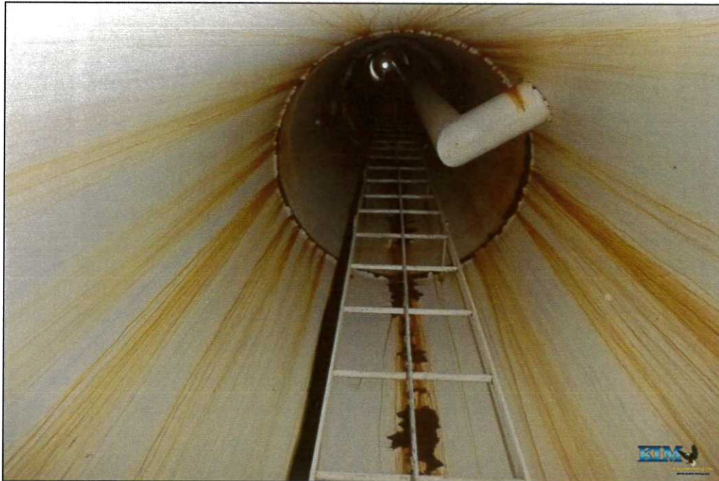
Photo No. 29 Condition of interior dry coating inside drywell tube Significant coating peeling and surface corrosion; staining from corrosion areas
