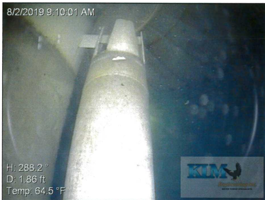
Photo No. 6 Condition of top of overflow pipe; view from below HWL
