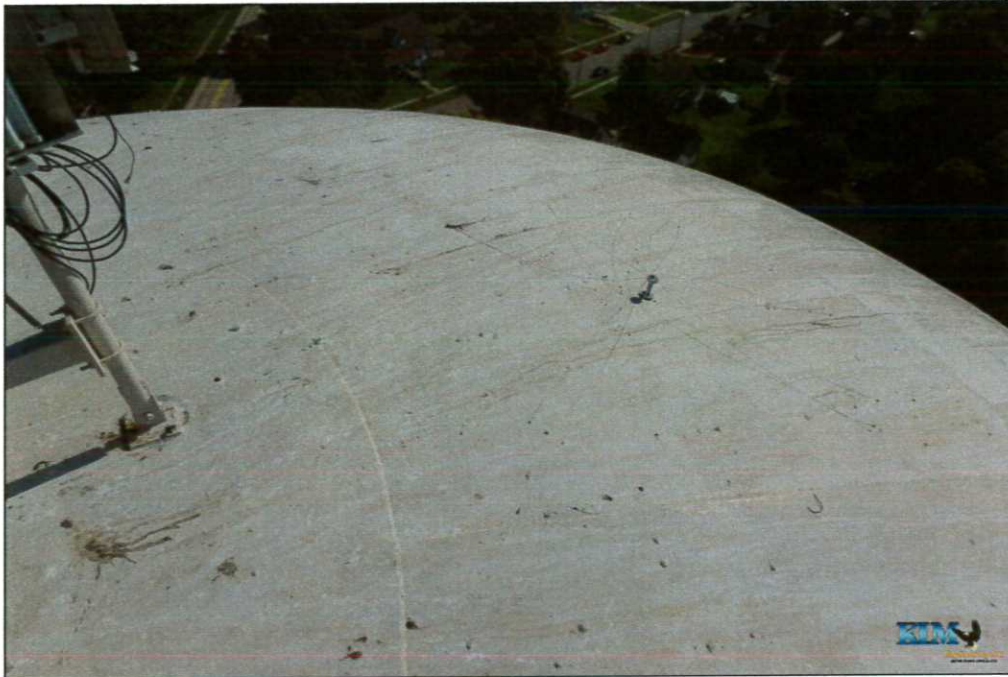
Photo No. 55 Condition of exterior coating on roof Bird droppings covering roof; non-functional bird deterrent visible
