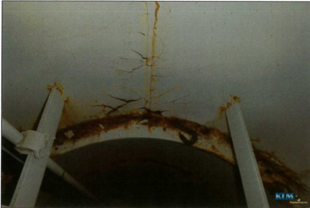
Photo No. 25 Condition of interior dry coating inside drywell tube Significant coating peeling and surface corrosion
