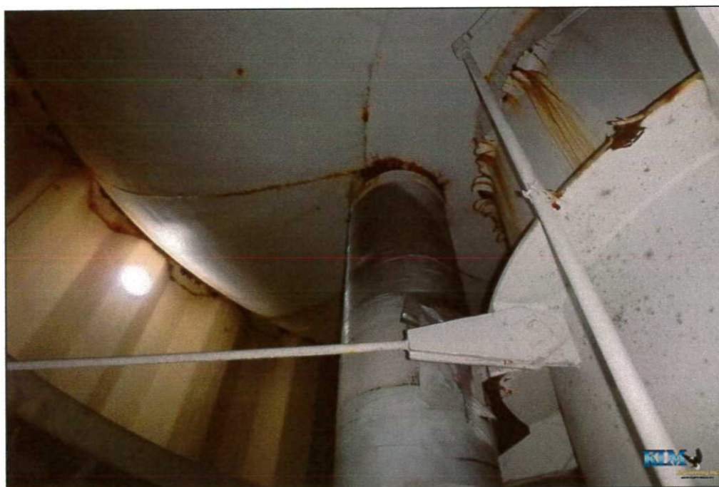
Photo No. 32 Condition of interior dry coating on bowl, drywell tube, fill pipe connection, and upper wall Random locations of heavy coating peeling and surface corrosion
