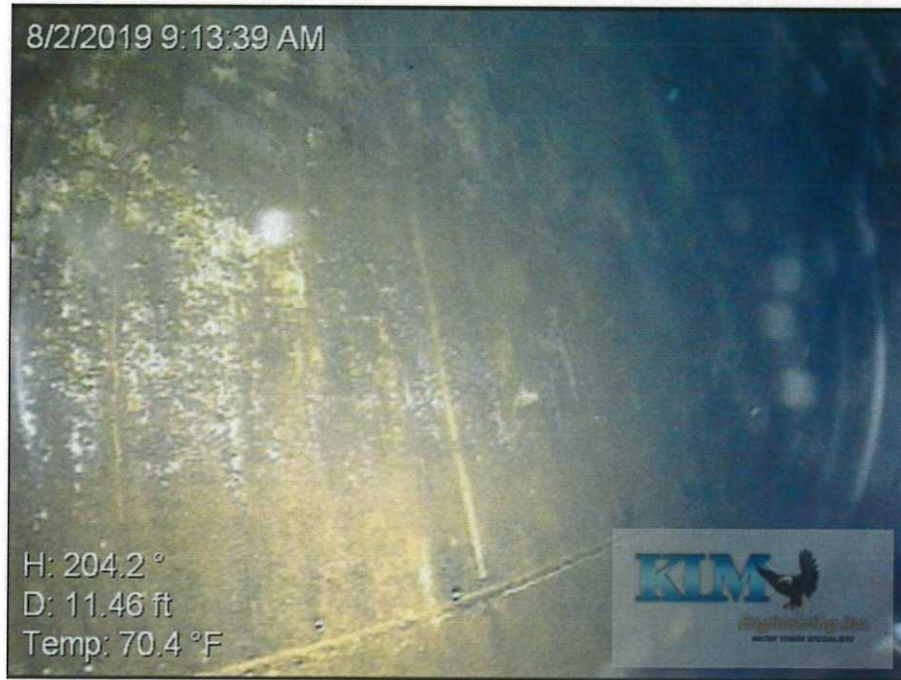
Photo No. 13 Condition of interior wet coating on shell wall Heavy staining and scale development
