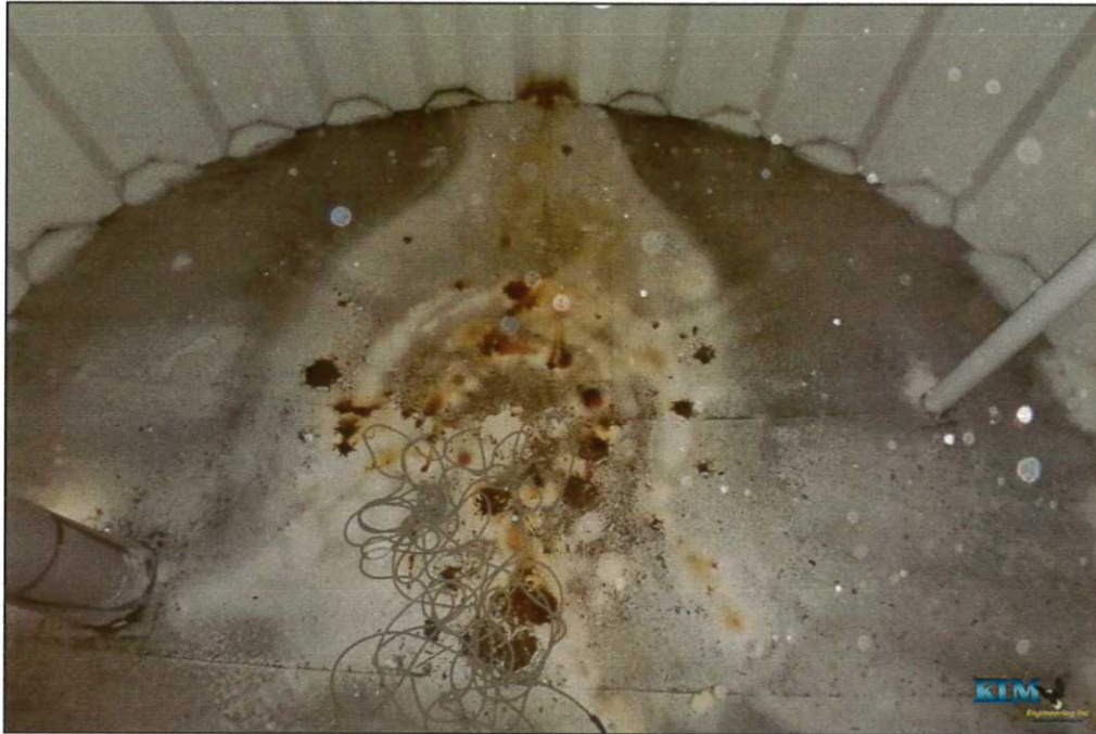
Photo No. 41 Condition of interior dry coating on condensate platform
