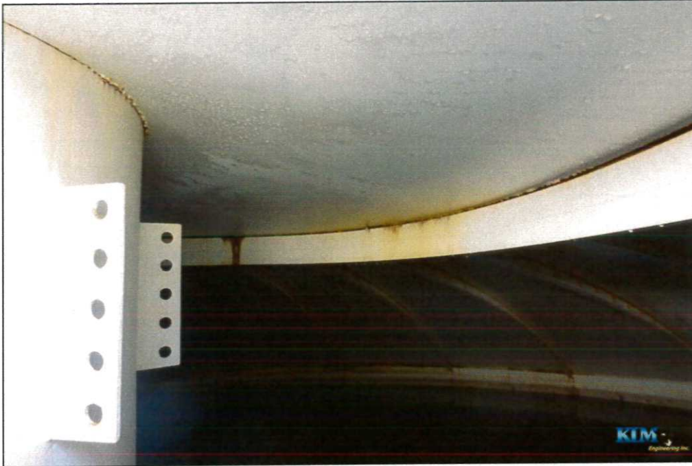
Photo No. 3 Condition of interior wet coating on roof around compression ring
