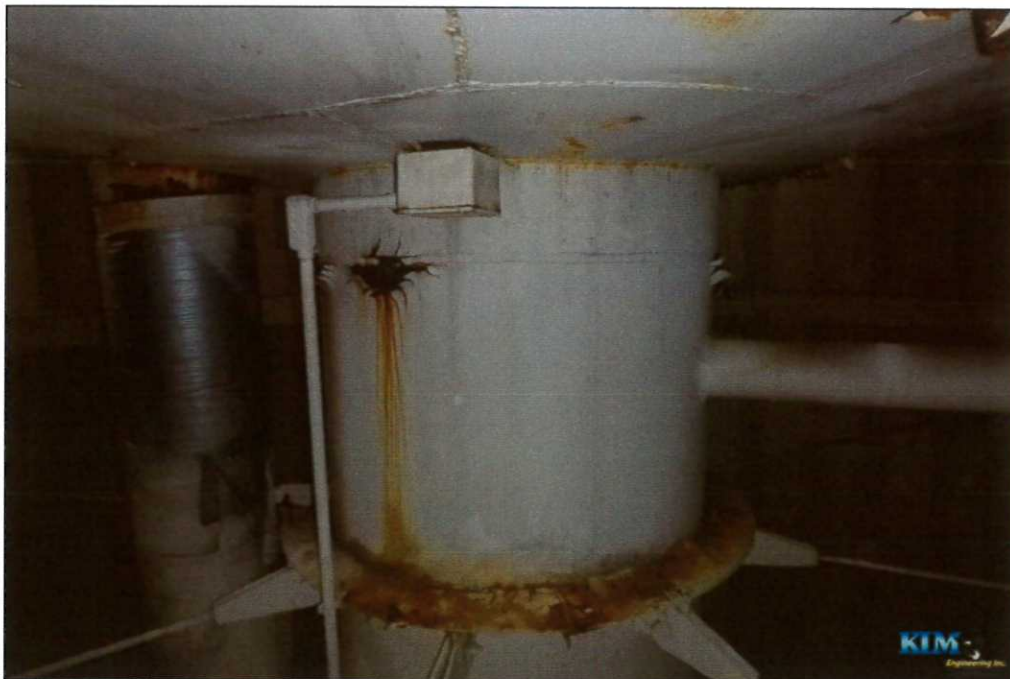
Photo No. 34 Condition of interior dry coating on drywell tube Cathodic protection system conduit and junction box visible
