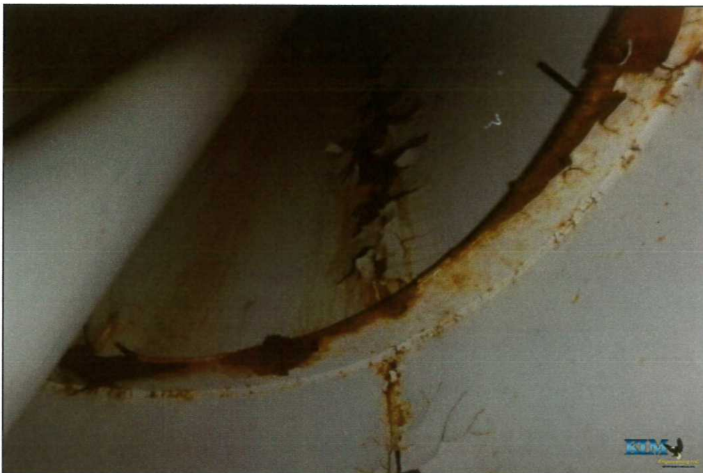
Photo No. 26 Condition of interior dry coating inside drywell tube Significant coating peeling and surface corrosion
