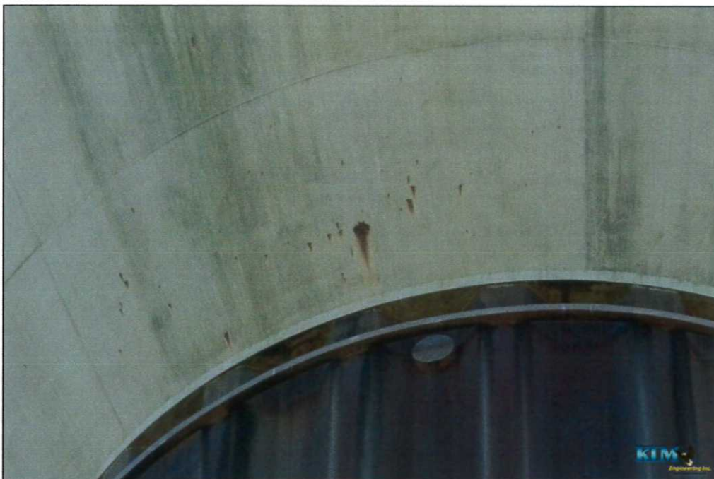
Photo No. 58 Condition of exterior coating near base of tank Spot and surface corrosion visible
