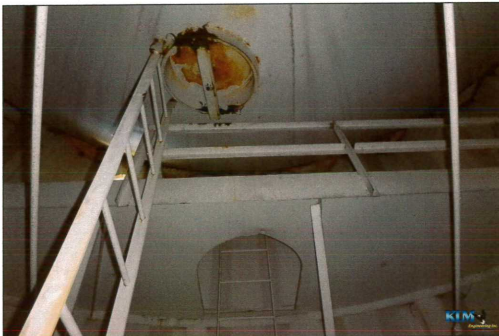
Photo No. 31 Condition of interior dry coating on bowl at bowl manway Random locations of heavy coating peeling and surface corrosion
