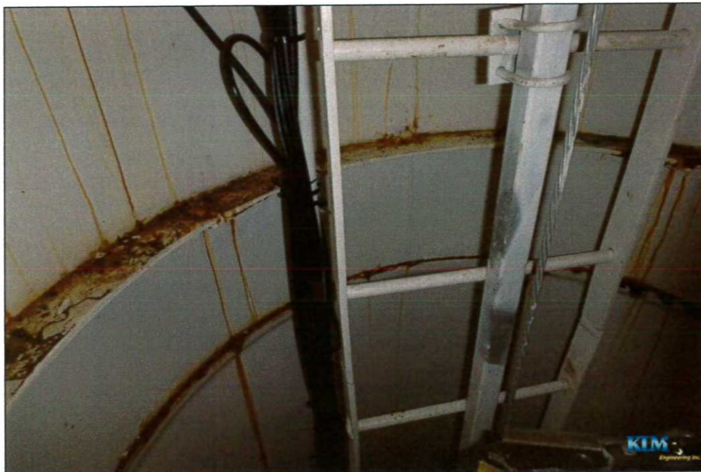
Photo No. 24 Condition of interior wet coating inside drywell tube
