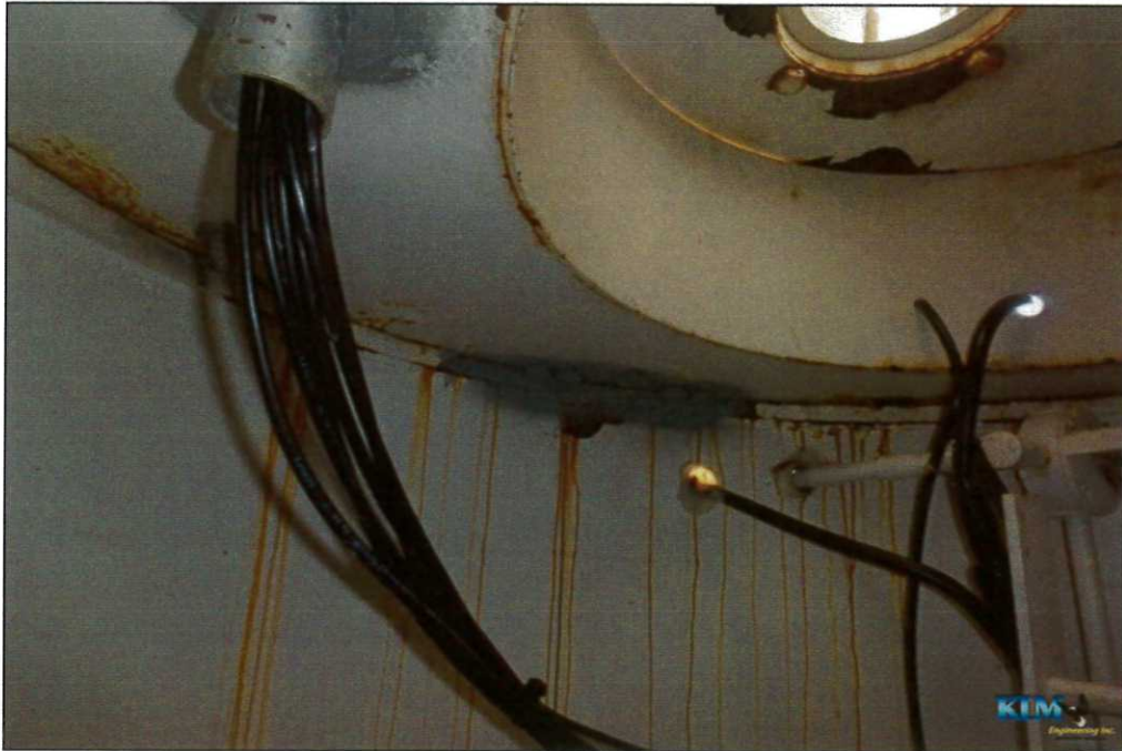
Photo No. 21 Condition of interior dry coating at top of drywell tube Significant peeling and surface corrosion occurring
