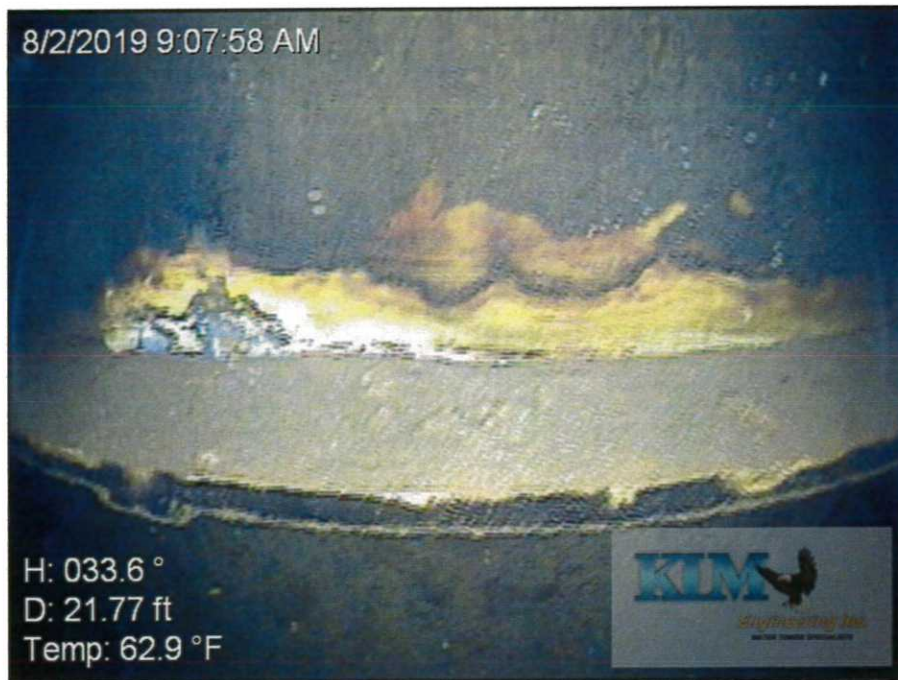
Photo No. 8 Condition of interior wet coating on drywell tube at stiffener ring Rust coloration due to corrosion
