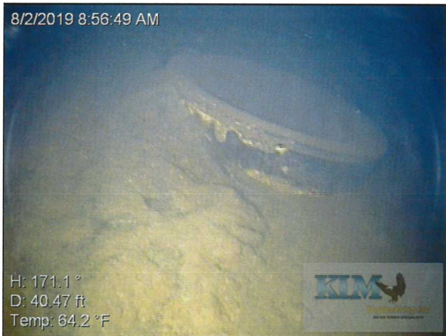
Photo No. 18 Heavy sediment accumulation and scale deposits in bowl Bowl manway visible
