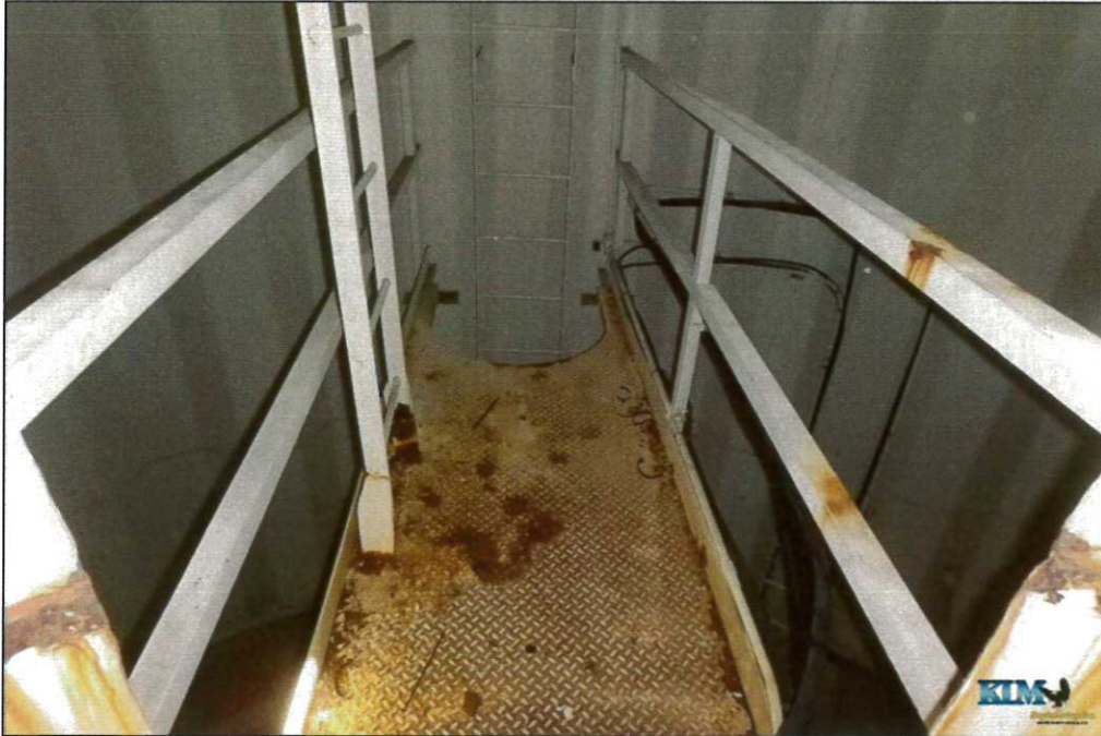
Photo No. 37 Condition of interior dry coating on drywell tube platform
