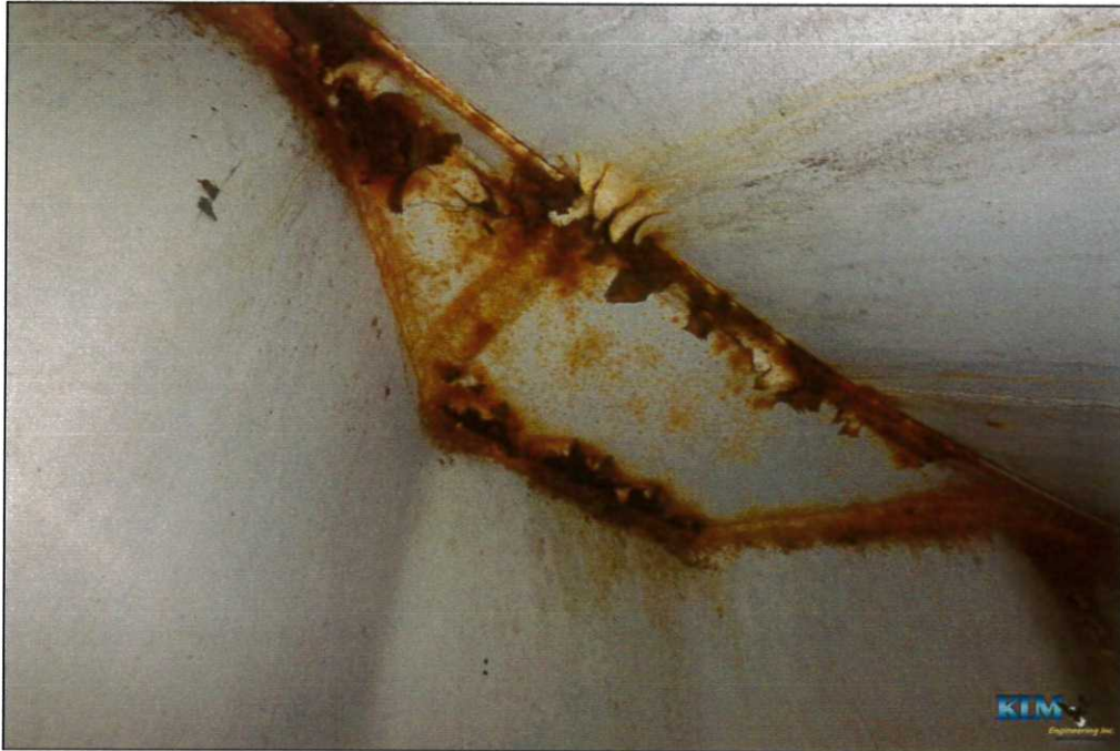
Photo No. 33 Condition of interior dry coating on bowl to wall connections
