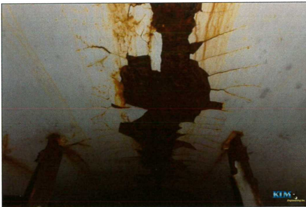
Photo No. 28 Condition of interior dry coating inside drywell tube Significant coating peeling and surface corrosion
