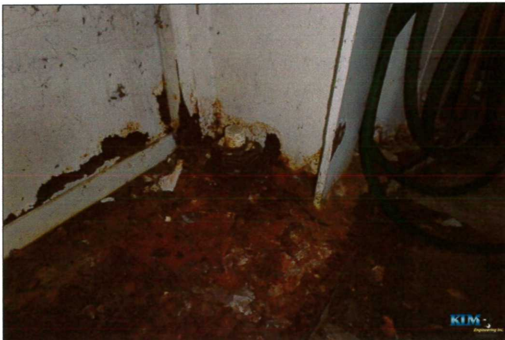
Photo No. 48 Condition of interior wet coating at base pedestal at double access doors Severe corrosion occurring on doors and on door frame
