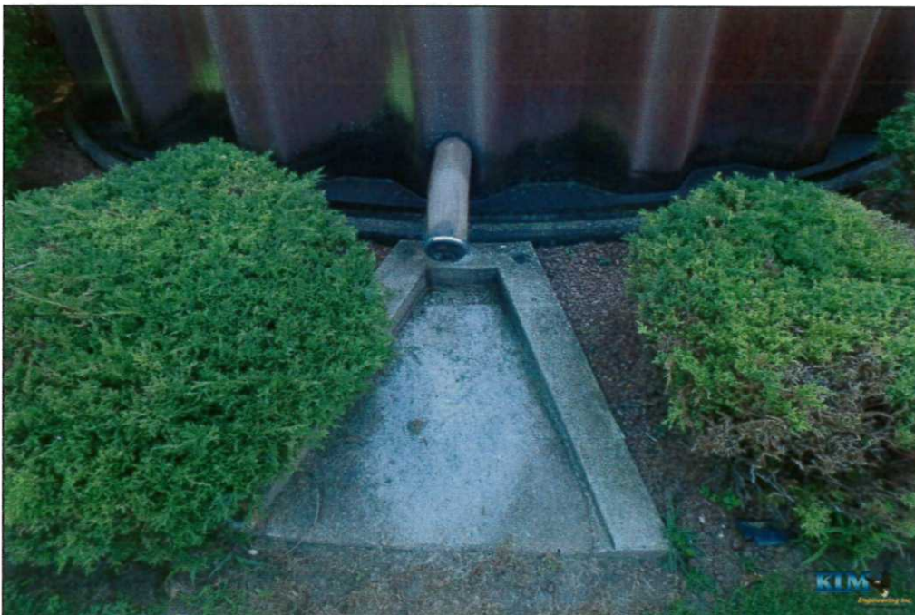
Photo No. 62 Condition of overflow pipe and splash pad at base of tower
