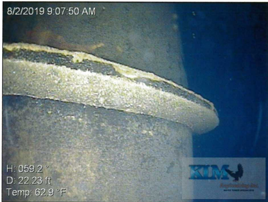
Photo No. 9 Condition of interior wet coating on drywell tube at a stiffener ring
