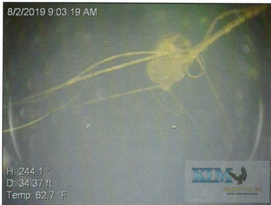
Photo No. 14 Submerged cathodic protection system
