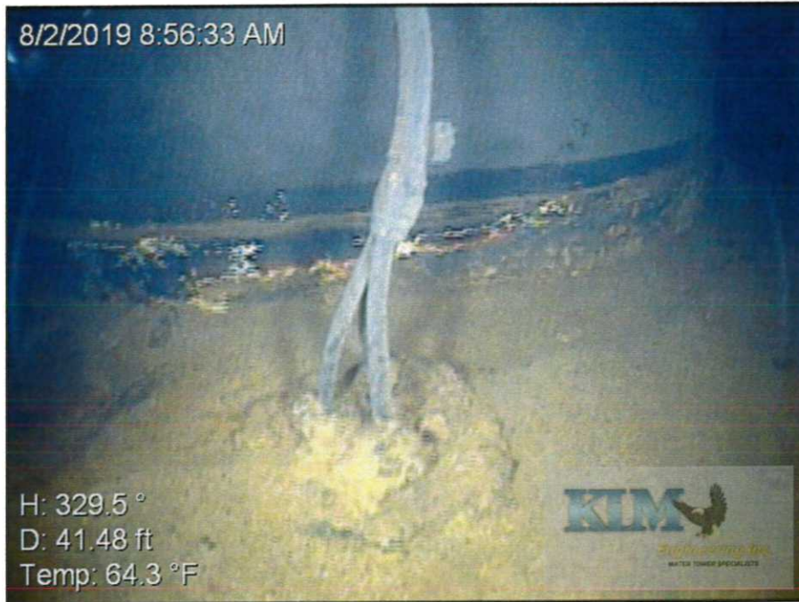
Photo No. 19 Condition of interior wet coating at base of drywell tube Cathodic protection cables visible
