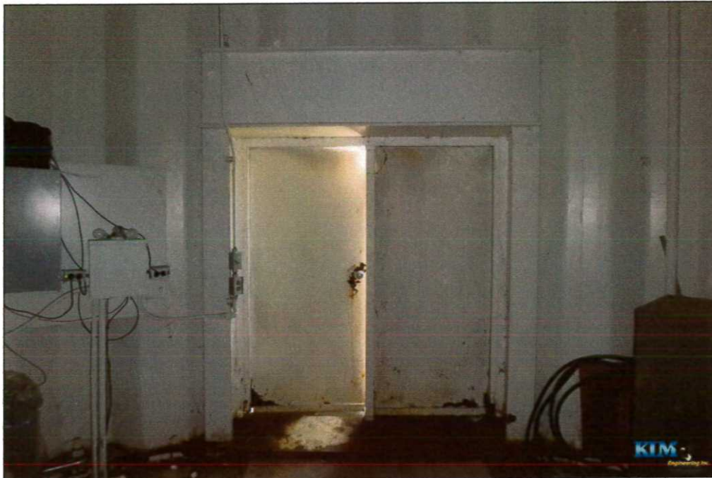
Photo No. 47 Condition of double access doors at base of pedestal Doors are severely corroded in bottom corners
