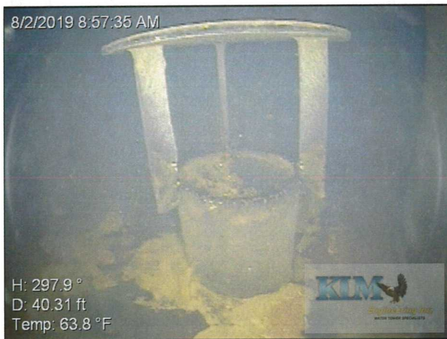
Photo No. 20 Condition of fill pipe in bowl Sediment accumulation visible around pipe
