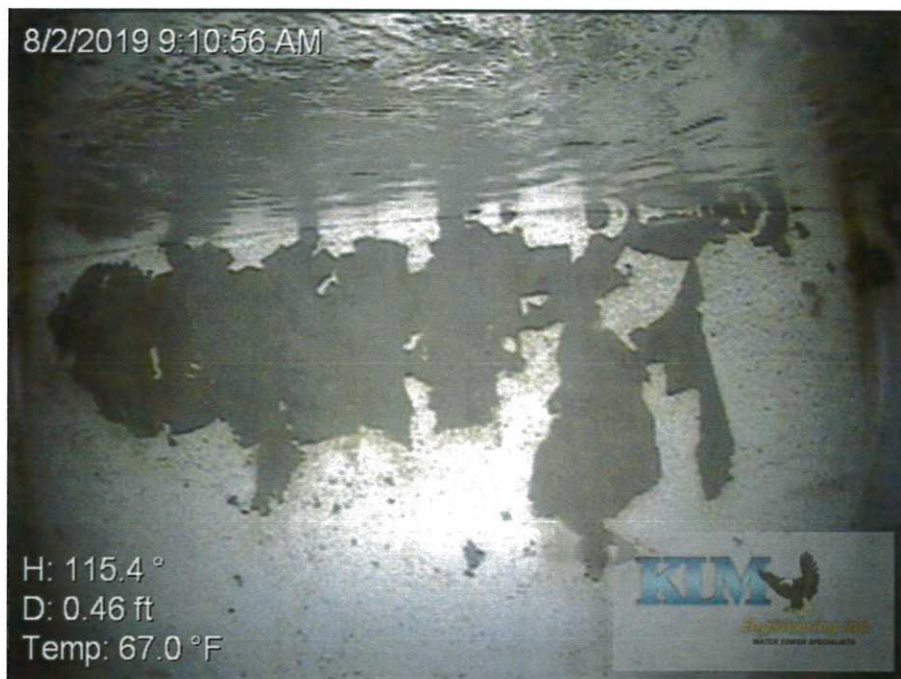
Photo No. 10 Condition of interior wet coating just below HWL Dark scale formation on shell
