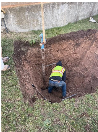
Picture 1.9 – Four of the non potable hydrants that we use for cleaning at the wastewater plant were replaced because the original ones were cracked and leaking.
