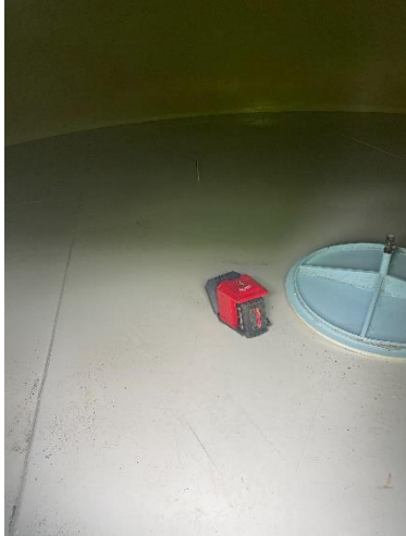
Picture 1.2 – The inside of the standpipe while the mixer was being installed.
