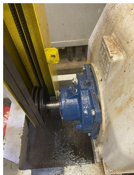
Picture 1.8 – The main lift station pump #1 had the impeller and drive assembly completely replaced.
