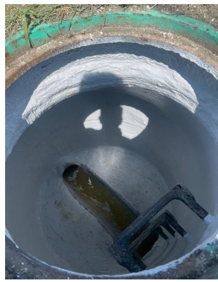
Picture 1.11 – Great Lakes relined a crumbling manhole located on Hwy-42 with a protective coating to prevent hydrogen sulfide gas damage.
