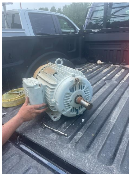
Picture 1.6 – 25 hp aeration drive motor that was replaced with the help of Energenecs in 2023.
