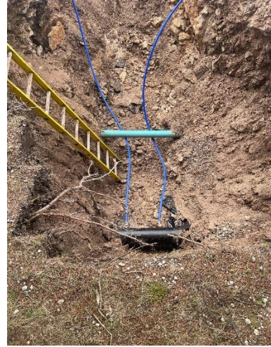
Picture 1.4 – A double water main tap done for curb stop placement located on Fieldcrest.
