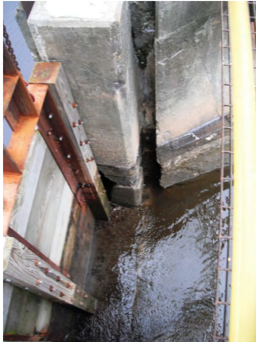
Degraded concrete near left control gate.
