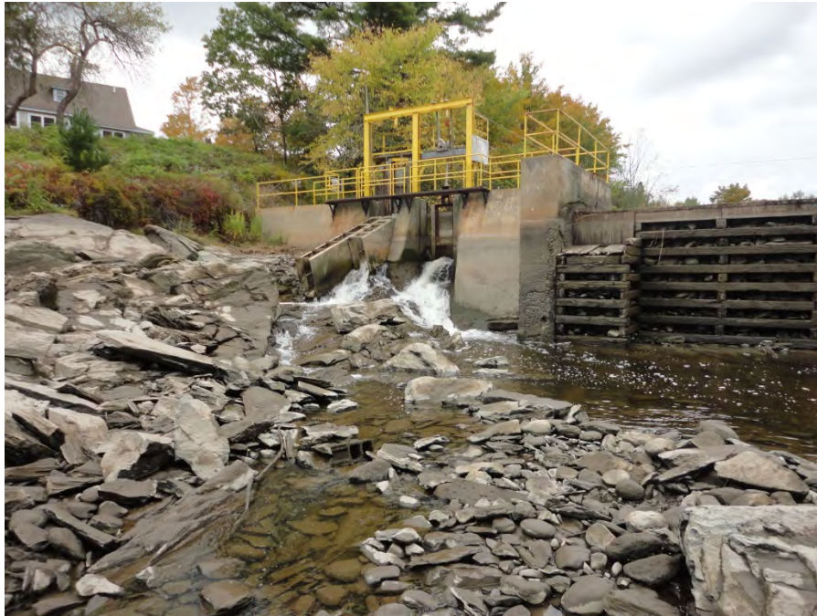
Control gates and fishway sections, low tide – fishway non-operational, non-functional.
