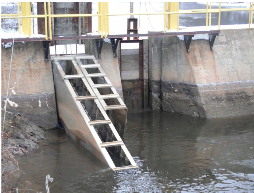
Control gates and fishway sections, middle of the tide – fishway non-operational, non-functional.
