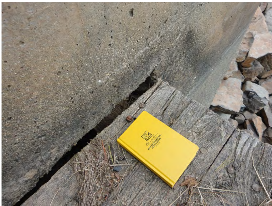
Spillway separation from left concrete abutment.
