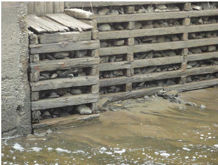
Seepage under/through dam.
