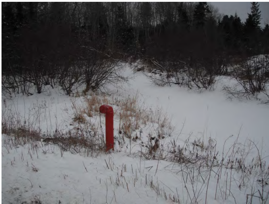
Dry hydrant on State Route 46 (White's Brook).
