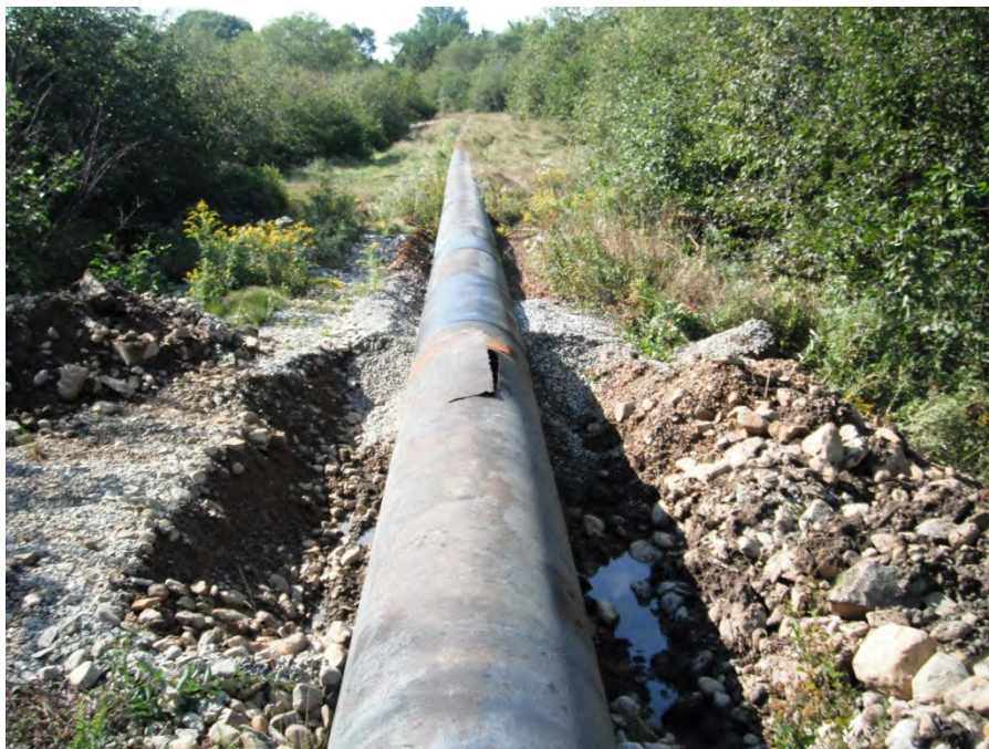
The Verso Corporation water diversion aqueduct. A “water hammer” ruptured pipe in 2012.
