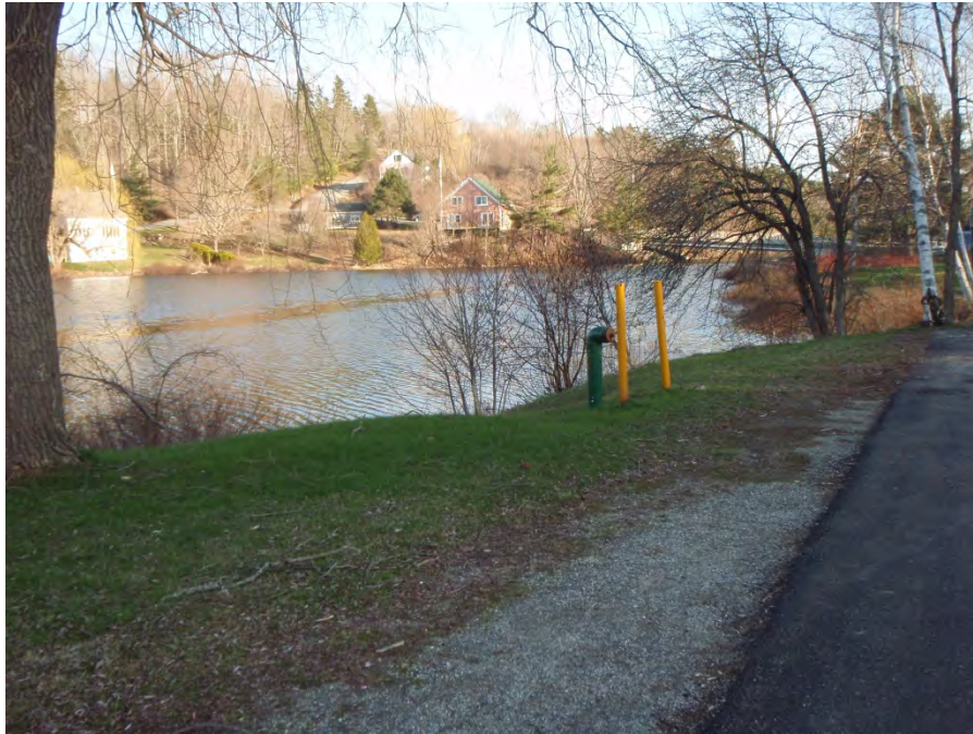
Dry hydrant on Narramissic Drive (impoundment).
