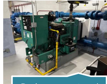
Backup generator w/ new electrical controls
