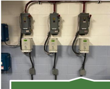
Booster Pump Controls
