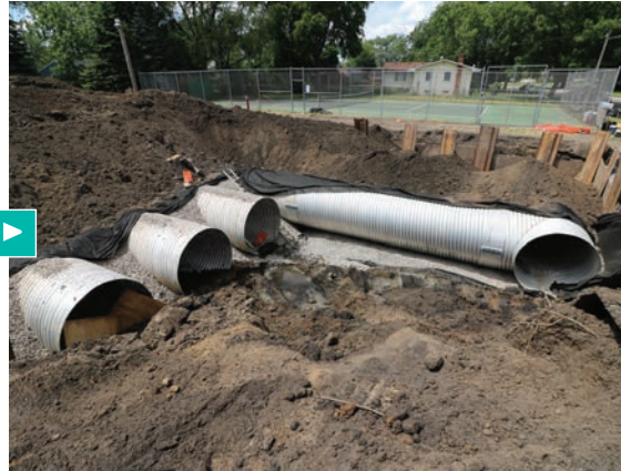
An underground stormwater infiltration system under construction at a park in Minneapolis. (Photo credit-"Infiltration System" by Mississippi WMO is licensed under CC BY-NC 2.0).
