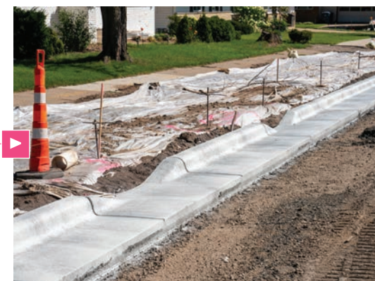
Construction of tree trench in Hoyer Heights, Minneapolis. (Photo credit- "Hoyer Heights Tree Trenches" by Mississippi WMO is licensed under CC BY-NC 2.0).
