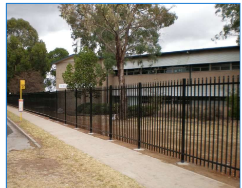
After: Freemont Elizabeth. 2100mm high security fencing dramatically increases the security of the site.
