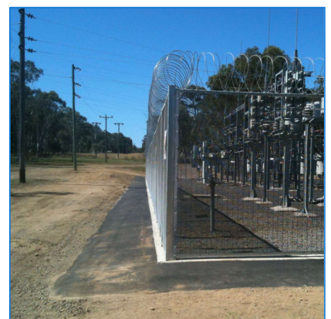
Fencing finished and asphalt placed around the perimeter of the site for earthing purposes (Coonabarabran)
