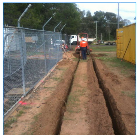
Excavation of earth grading ring around the outside of the zone substation (Coonabarabran)
