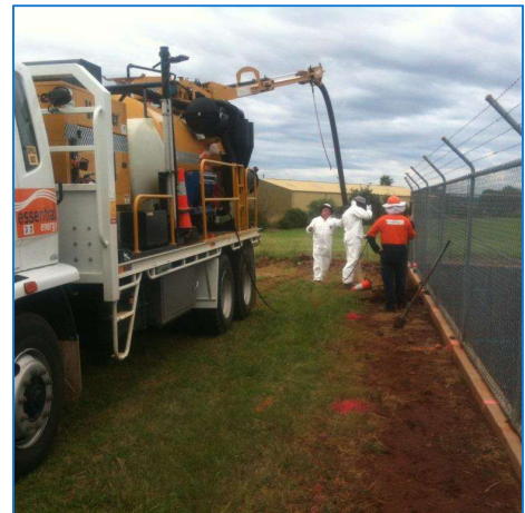
The use of water vacuum excavation to locate optic fibre in close vicinity to the new fence line (Dubbo)
