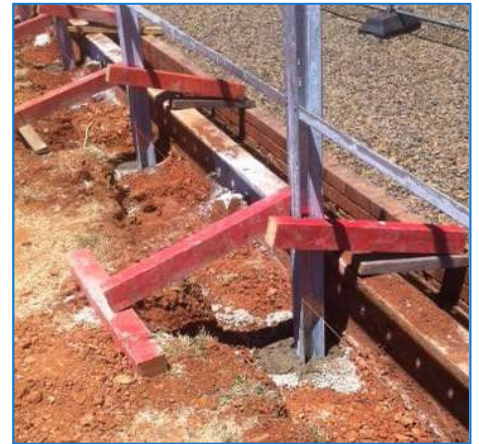
Intermediate channel posts are set to height, in line and plumb by adjusting the timber jigs.
