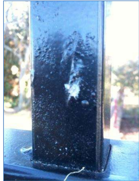
An example of delamination (failure) of the powder film. This is likely a result of contaminants or oxidation (white rust) on the surface of the steel before coating. This image was taken less than 18 months after installation of the fence.
