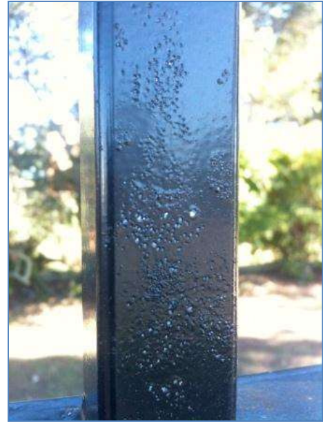
An example of 'pin holing' most likely a result of low quality powders and/ or poor pretreatment and cleaning of the steel surface before coating. This image was taken less than 18 months after installation of the fence.
