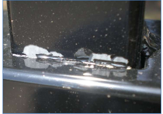
An example of the powder film delaminating as a result of poor metal pretreatment and under cure. This image was taken less than 1 month after installation of the fence.
