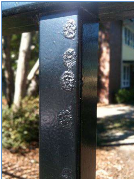
An example of blistering of the powder coating or the 'orange peel' effect a result of poor quality metal surface preparation on an imported panel. This image was taken less than 18 months after installation of the fence.
