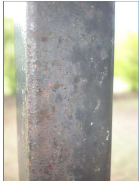
A close up of image (left) showing failure of the powder coating at 24 months. The film has severely faded and lost its barrier corrosion protection qualities.
