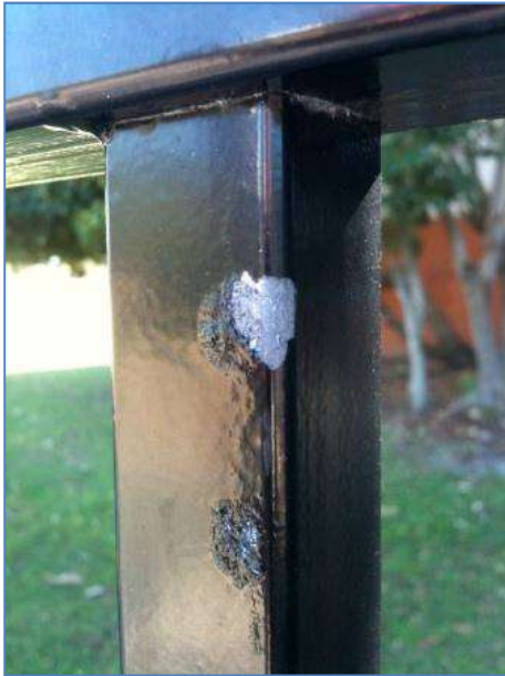
An example of delamination of the powder film. This image was taken less than 18 months after installation of the fence.
