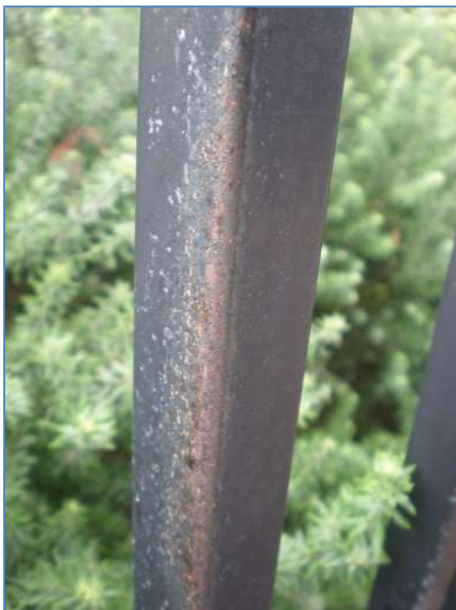
An example of the result of using low quality powder and insufficient coating thickness. The coating has severely faded. The coating has offered little barrier corrosion protection of the steel resulting in aggressive corrosion. This image was taken less than 24 months after installation of the fence.
