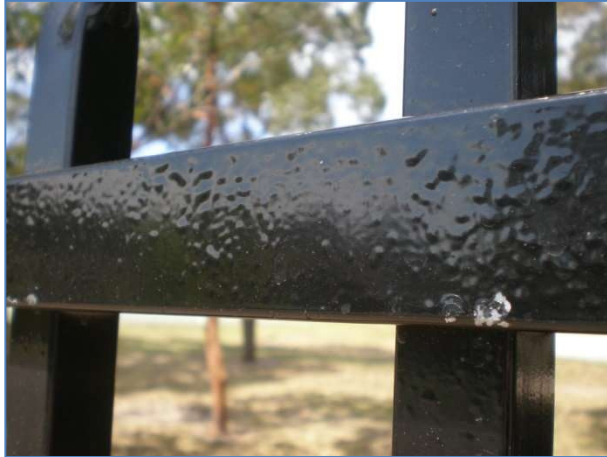
An example of the powder application being too 'heavy'. This powder film will be under cured and as a result the proper mechanical properties of the film will not have been achieved. The film will be 'soft' and will readily delaminate.
