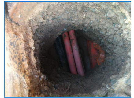
Contact with underground services was a constant threat and vacuum excavation was often used to expose detected services.
