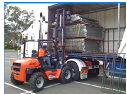
Unload of bulk materials on site from semi-trailer direct from our factory.
