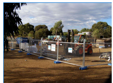
A site storage compound on site is often used to secure materials restrict access.
