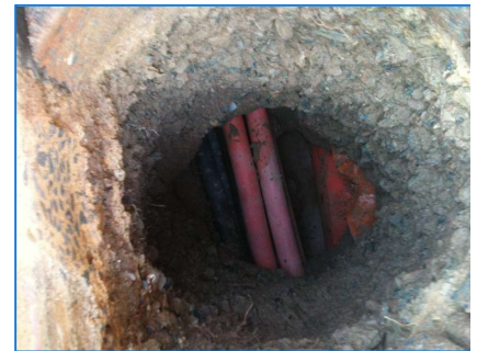
Contact with underground services was a constant threat and vacuum excavation was often used to expose detected services.
