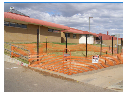
The schools are normally operational and therefore restricting access to the work area is critical.
