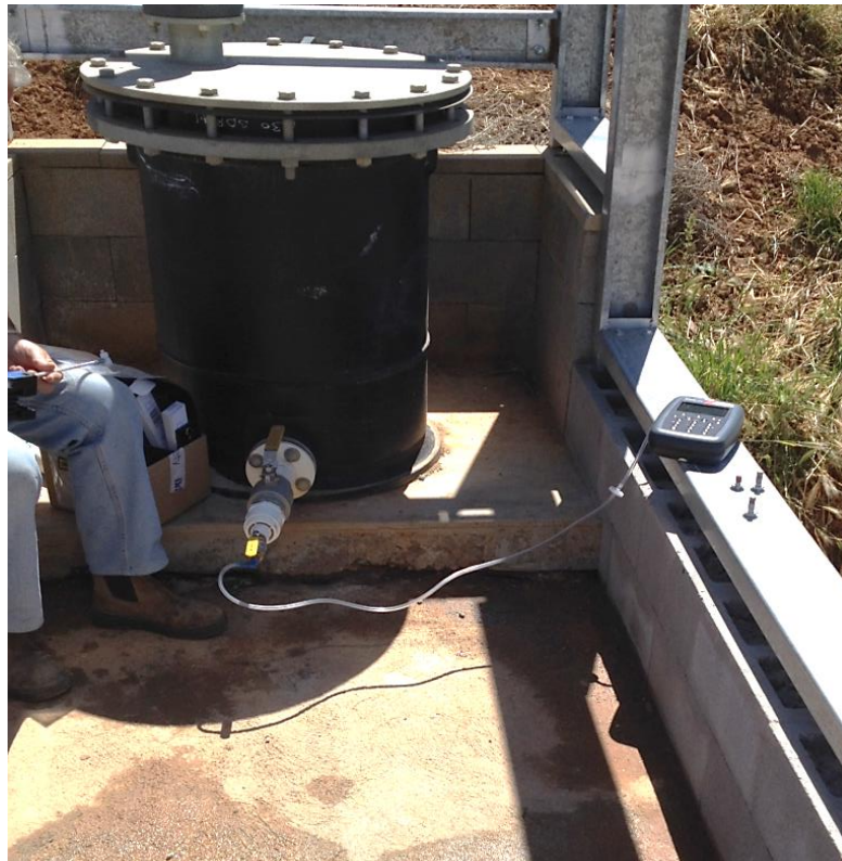
Figure 3.1 Measurement of biogas composition on-farm can confirm whether explosive gas mixtures have successfully been purged from biogas equipment and piping. The biogas meters shall be appropriately rated for use in potentially explosive gas atmospheres (courtesy of the Pork CRC)
