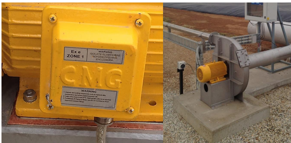
Figure 2.2 Example of a biogas blower at an Australian piggery rated to Zone 1 (Photos courtesy of the Pork CRC)
