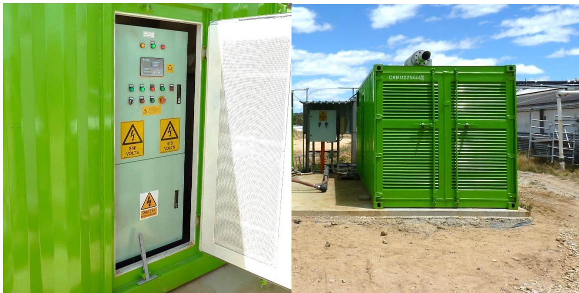
Figure 2.4 Emergency switches located outside an on-farm generator skid (Photos courtesy of the Pork CRC)
