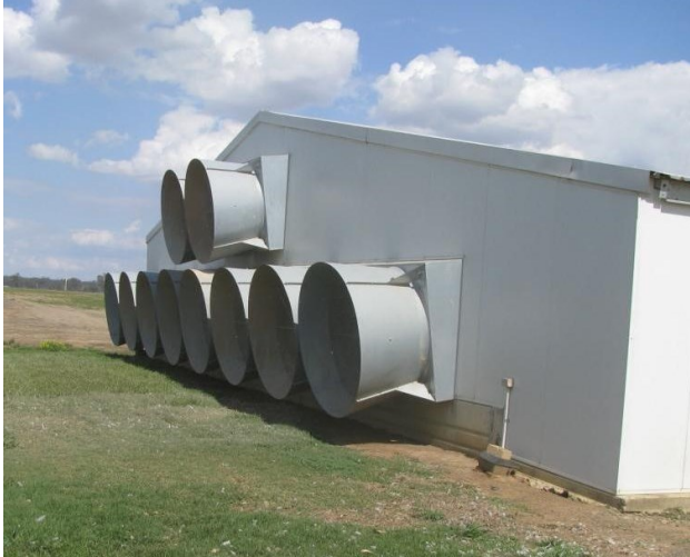
Photograph 7. Shed ventilation fans and discharge cones.
