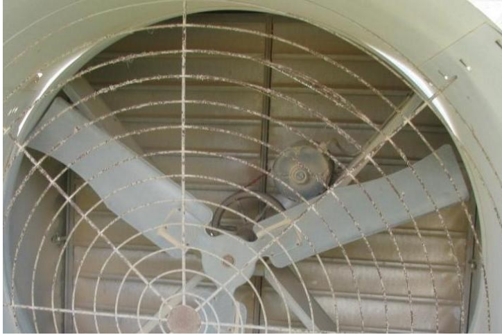
Photograph 8. Close up of ventilation fan showing three phase motor.
