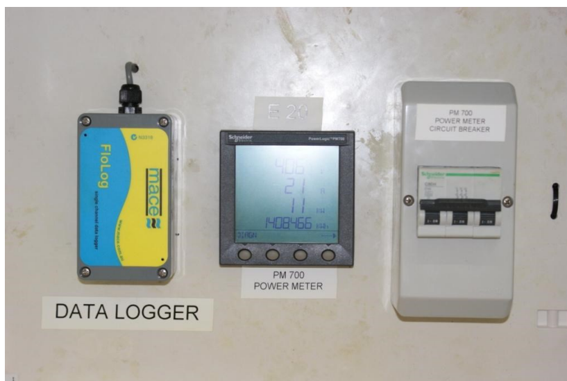
Photograph 6. Power meter and data logger installed in a poultry shed.
