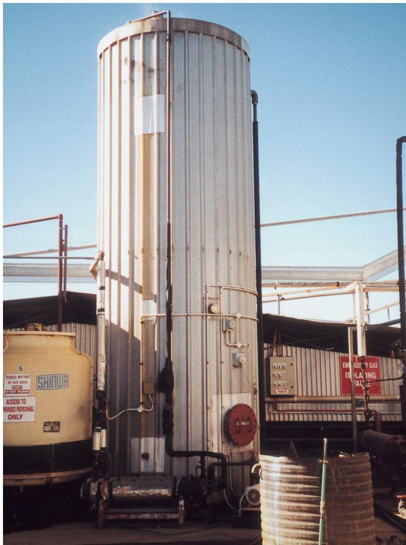
Hot water tank steriliser vat
