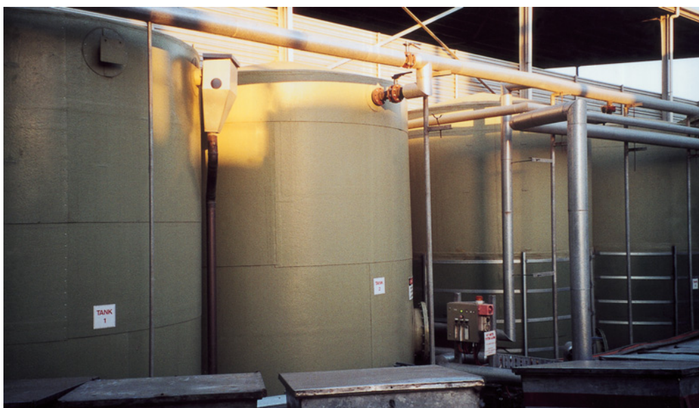
Water Chlorination tanks
